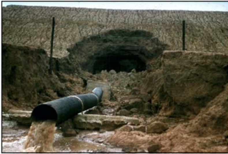
Figure 1 - "Piping" failure of a dam due to inadequate protective measures or construction methods.
