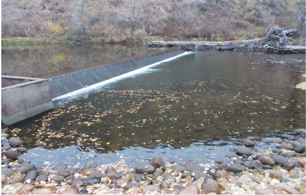
Jackson Ditch Diversion Dam on the Cache La Poudre River, Ft Collins, Colorado (Photo Courtesy of Wright Water Engineers)
