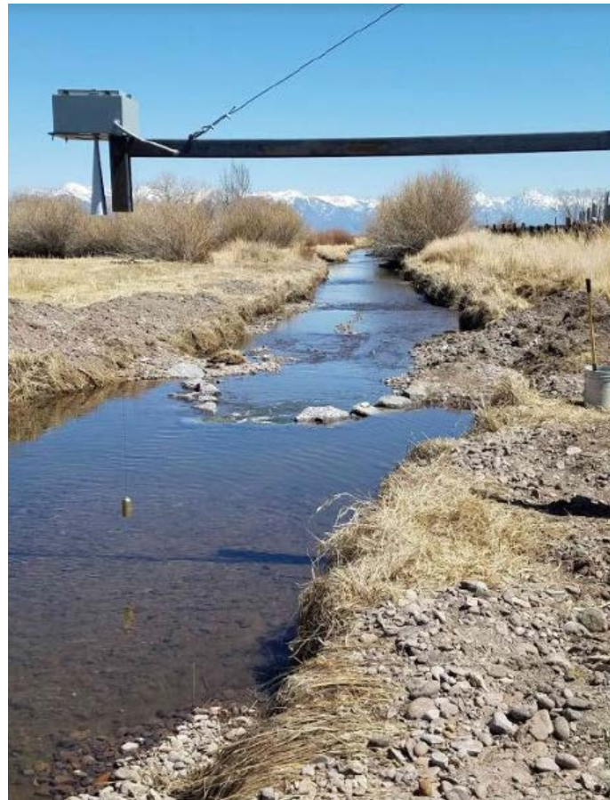
Saguache Creek at Cemetery Road- Cantilever and Radar Installation (Division 3). Note these installations are more cost efficient as they require significantly less infrastructure than a typical stilling well and shelter.
