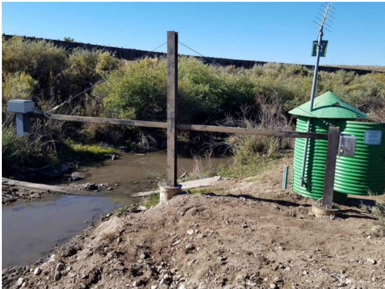
Trinchera Creek Below Smith Reservoir - Cantilever and Radar Installation (Note these installations are more cost efficient as they require significantly less infrastructure than a typical stilling well and shelter)
