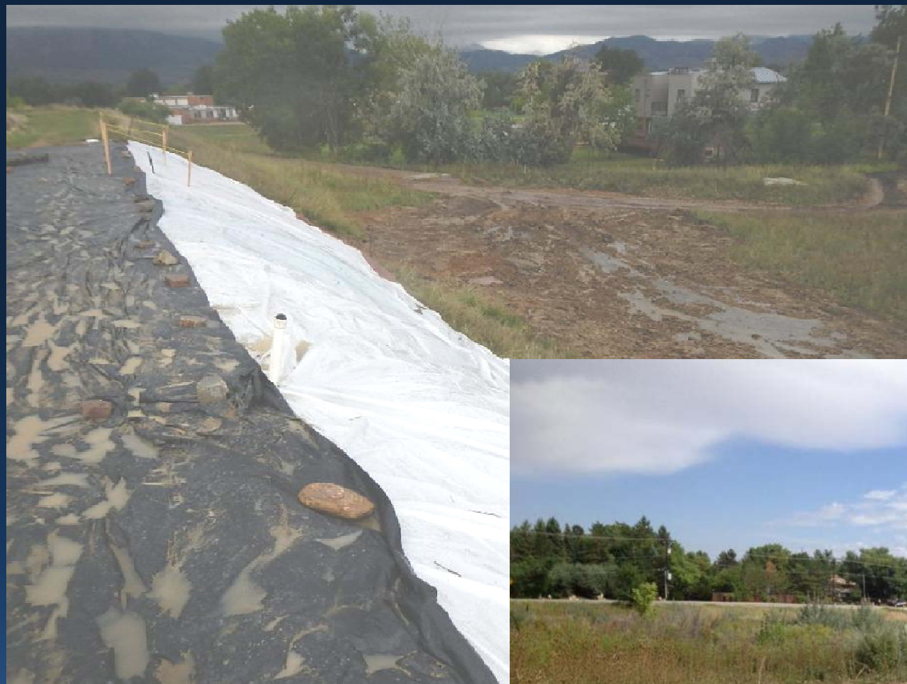
Baseline Dam Slope Buttressed
