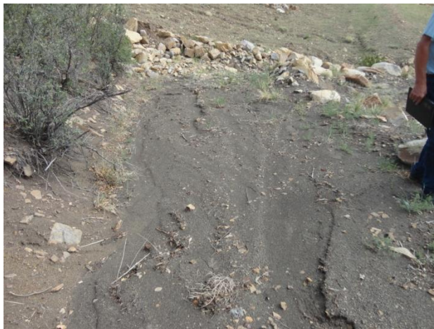
Photo 20: Contour ditch west of fill 7 to be cleaned (2)
