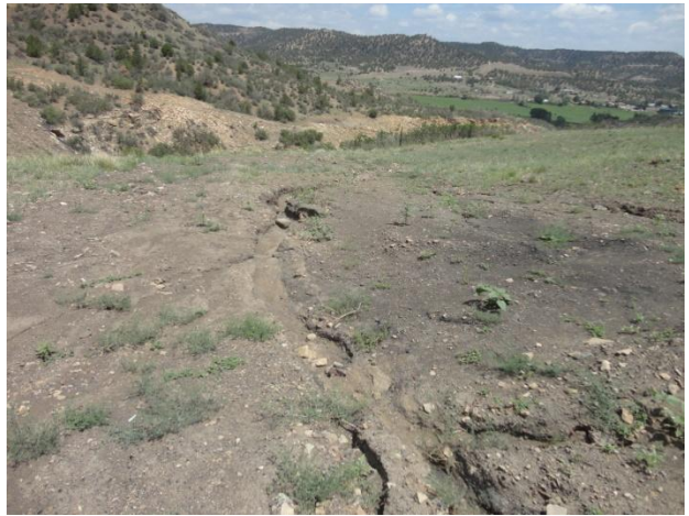
Photo 44: Erosion outside of fill 8 (1)
