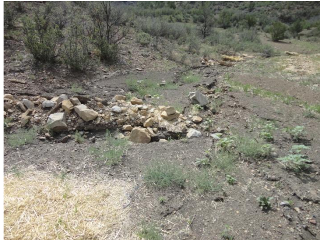
Photo 28: Erosion next to pond 6 emergency spillway (3)
