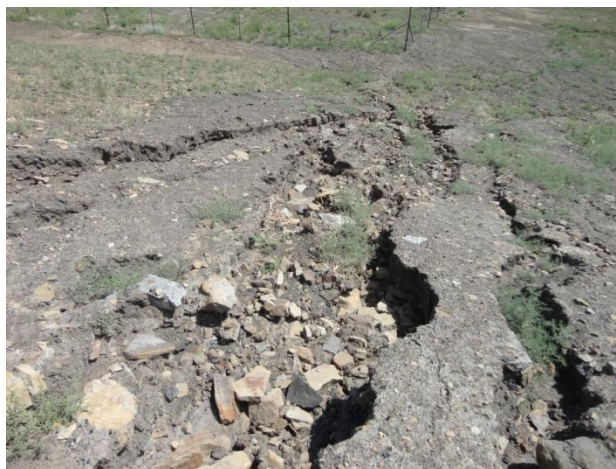
Photo 38: Close up of erosion in 37
