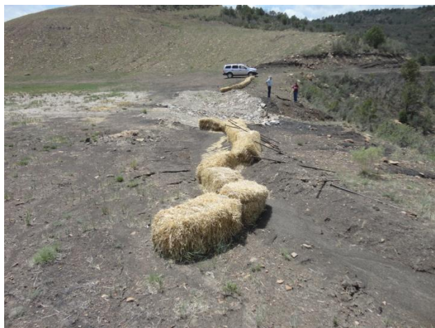
Photo 46: Flow control above pond 5
