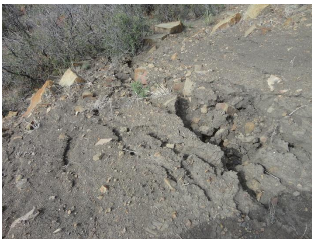
Photo 23: Erosion caused by breach shown in 22
