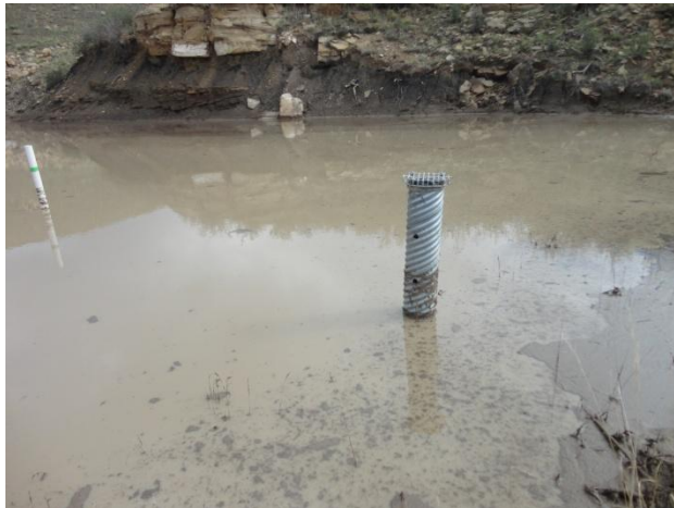
Photo 15: Pond 9A riser
