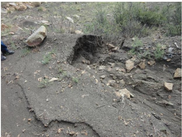
Photo 21: Erosion caused by breach of ditch shown in 19 & 20
