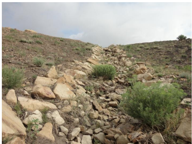
Photo 11: Excellent east down-drain on fill 9
