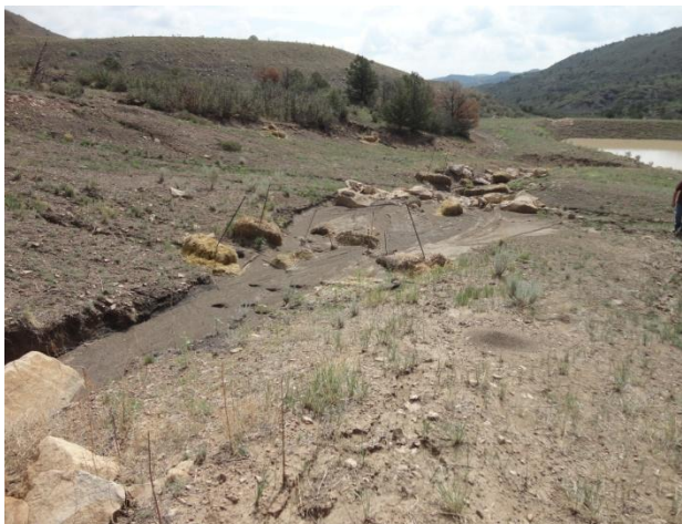
Photo 32: Accumulated sediment above pond 6 (3)
