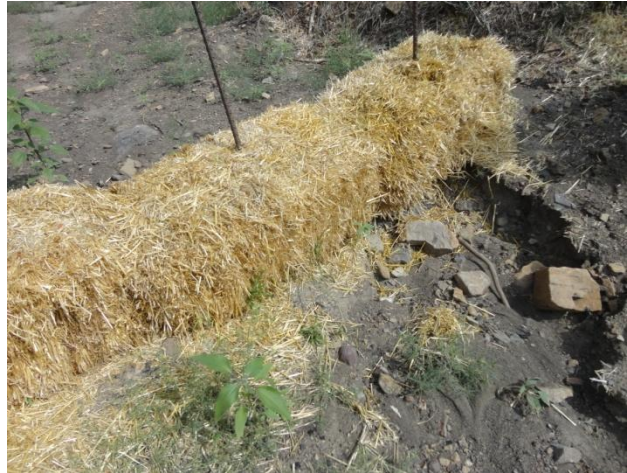
Photo 26: Erosion next to pond 6 emergency spillway (1)
