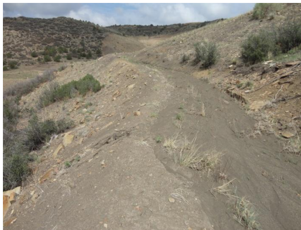
Photo 22: Breach of ditch between ponds 7 and 6
