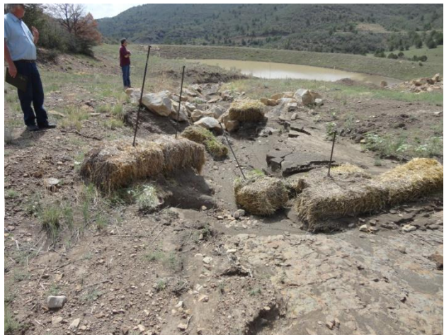
Photo 31: Accumulated sediment above pond 6 (2)
