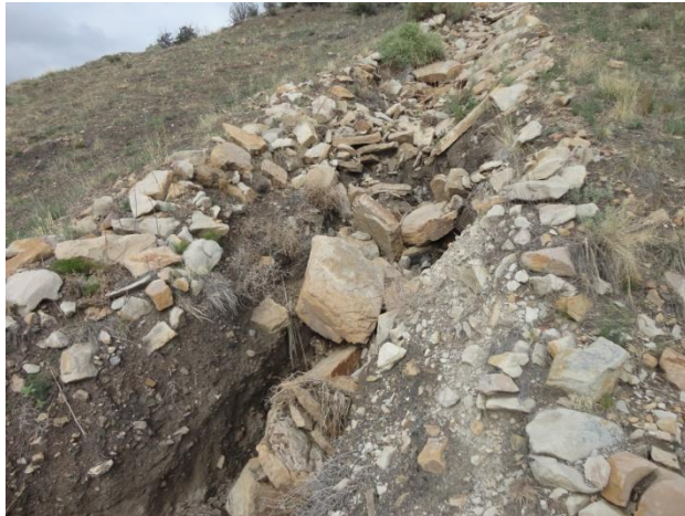
Photo 13: West down-drain on fill 9 needing repair (2)
