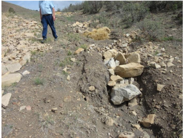
Photo 27: Erosion next to pond 6 emergency spillway (2)
