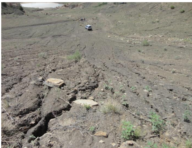
Photo 36: Steep slope above pond 6, showing erosion (3)
