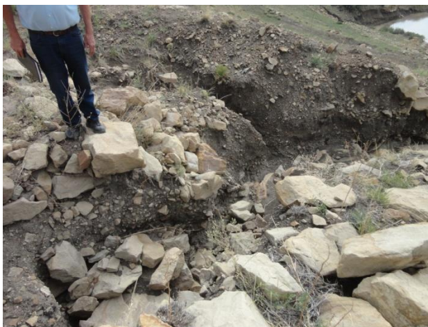
Photo 12: West down-drain on fill 9 needing repair (1)
