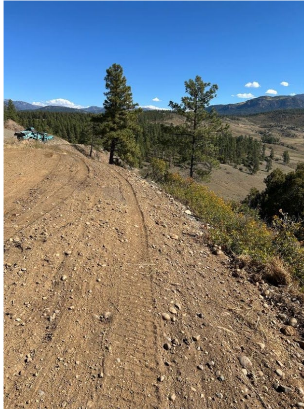
Photo 11: View affected land potentially outside of the approved affected area boundary on the east side within the Phase 3 area, facing north.
