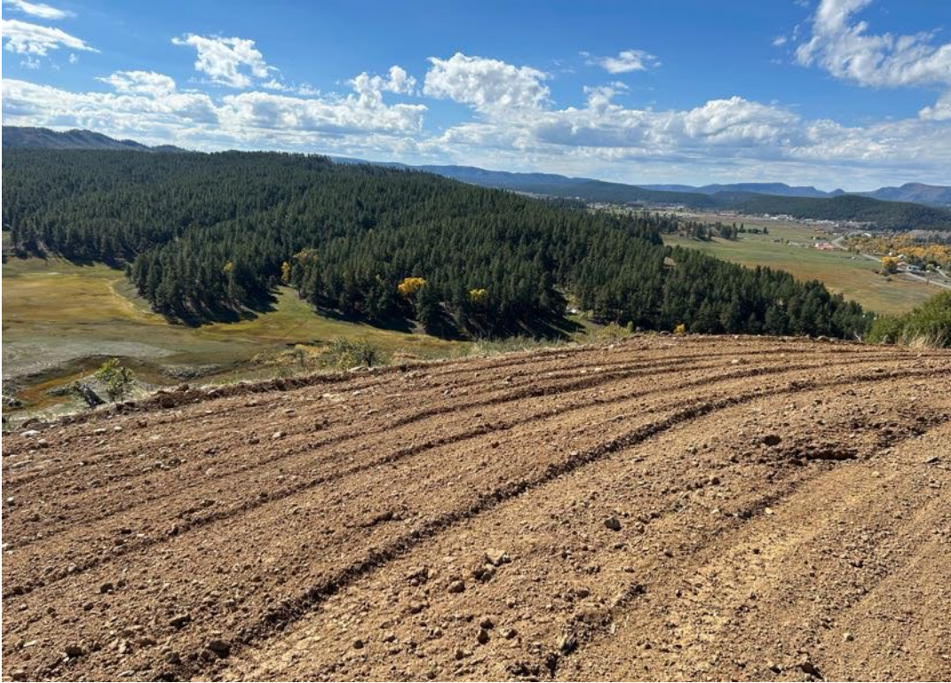
Photo 13: View of affected land potentially outside on the approved affected area boundary on the southern toe of the Phase 3 area, facing southeast.
