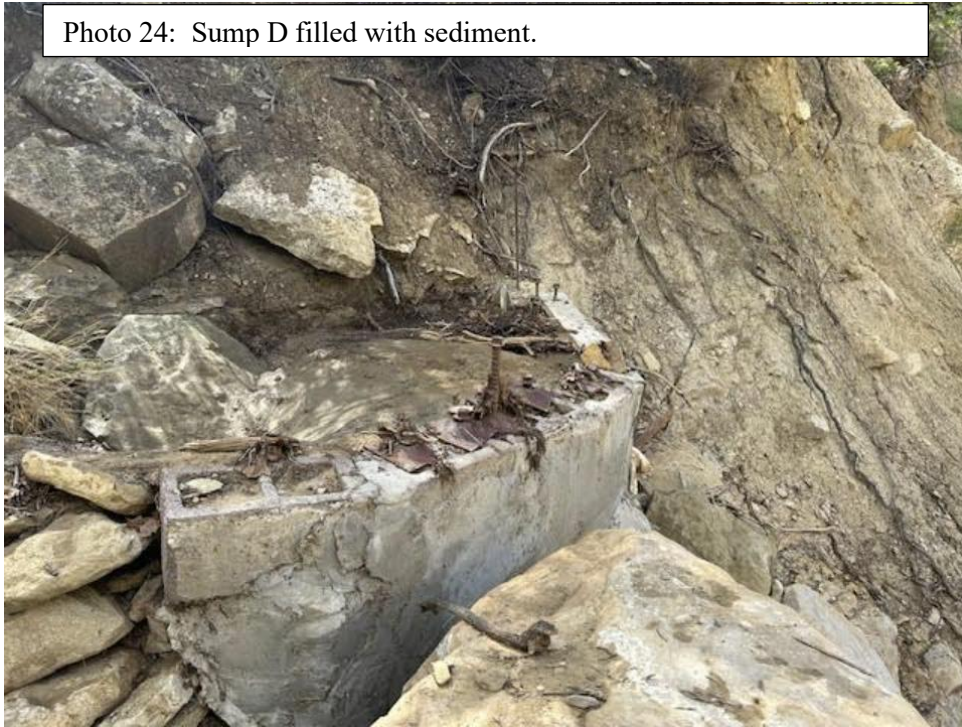
Photo 24: Sump D's embankment eroded, and the discharge pipe was exposed.
