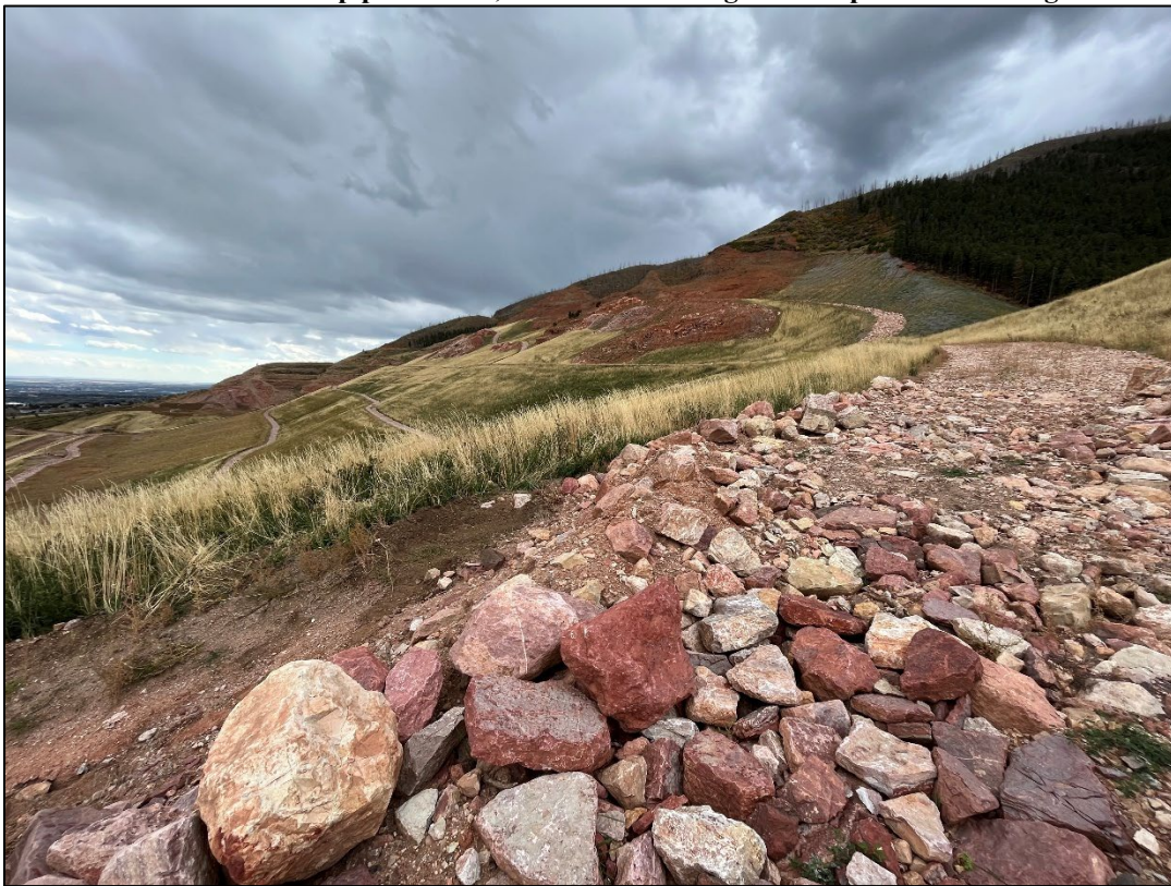
Photo 11: View southwest of the north channel, this area was observed to be the source of a few downslope erosional issues last inspection but has now been reformed to direct stormwater further into the channel.
