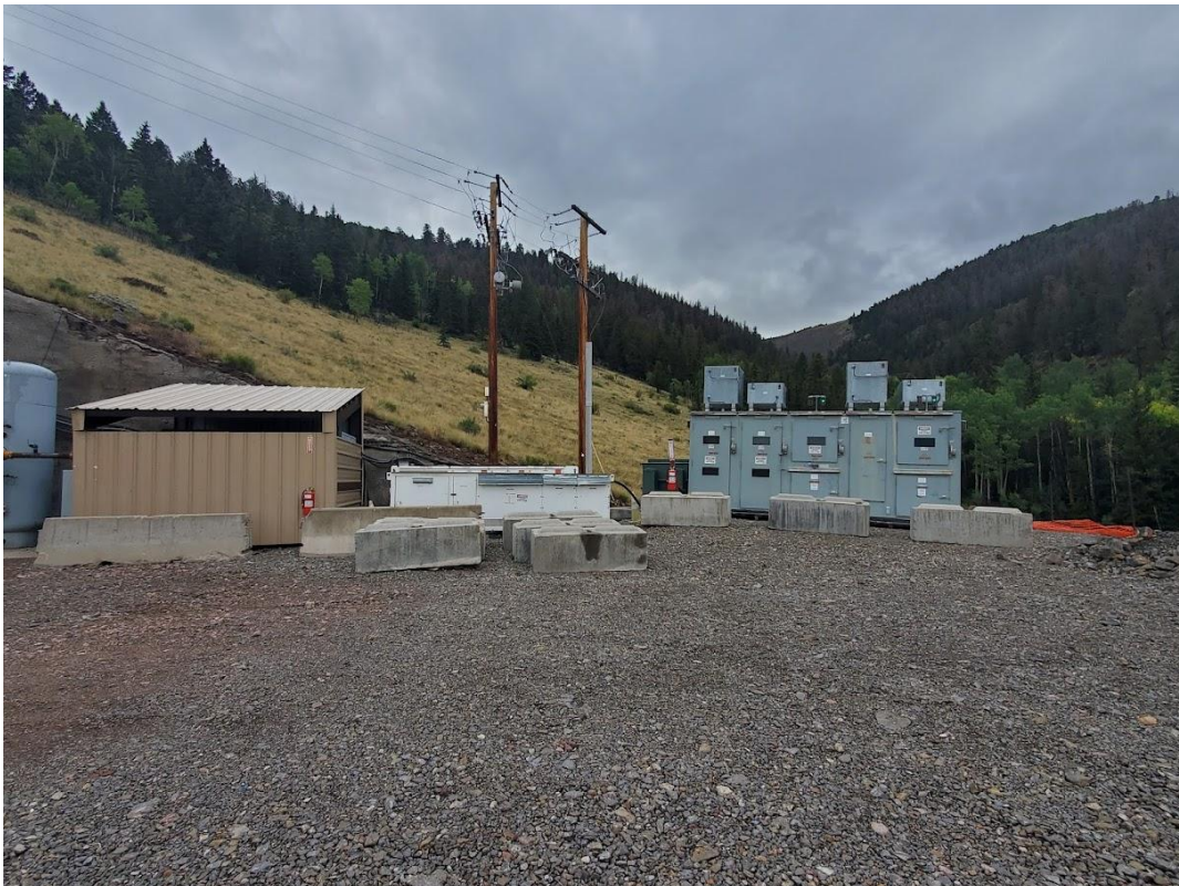
Photo 2: View to the north of electrical equipment at the 9400 Level Portal.
