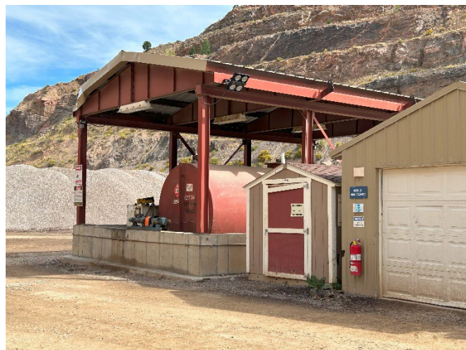
Photo 6: Diesel storage area. Note double lined containment.
