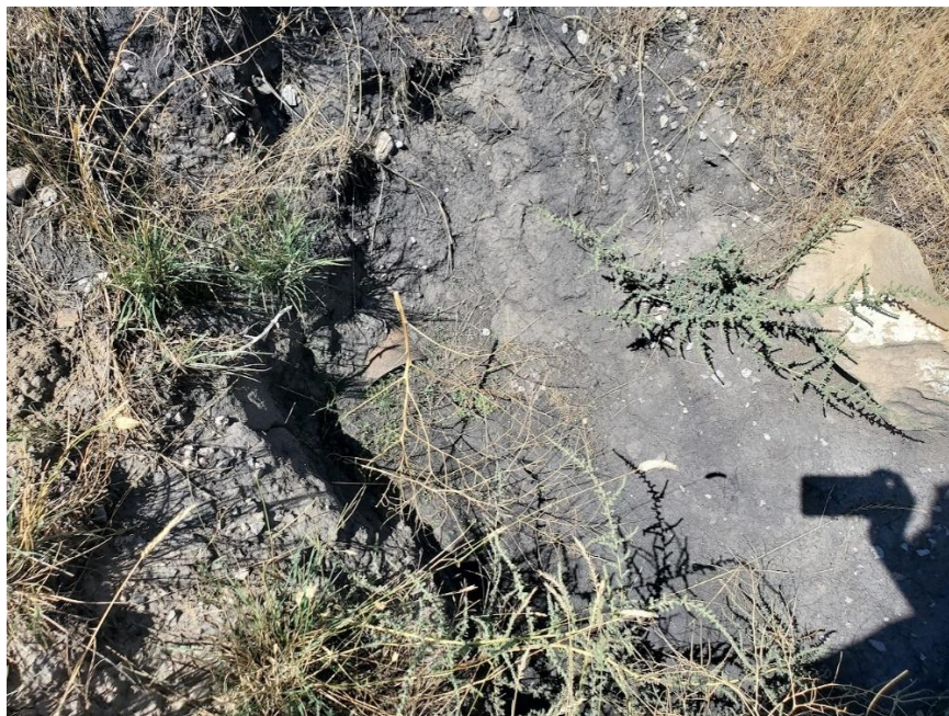
Photo 15: View to the south of culvert filled with sediment under the access road to the Nitrogen Injection Plant.
