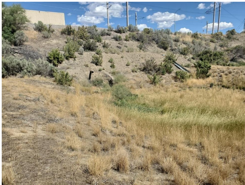
Photo 7: View to the north of the erosion scar in the RR-1 Pond.
