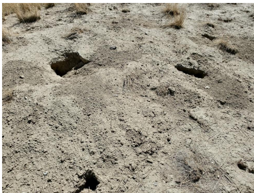
Photo 8: View to the south of animal burrows in the RP-4 Pond embankment.
