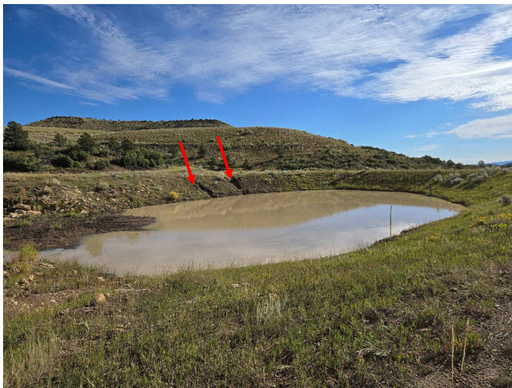
Photo 5: Looking northeast at Pond 006a. The arrow points to the erosion on the north bank.
