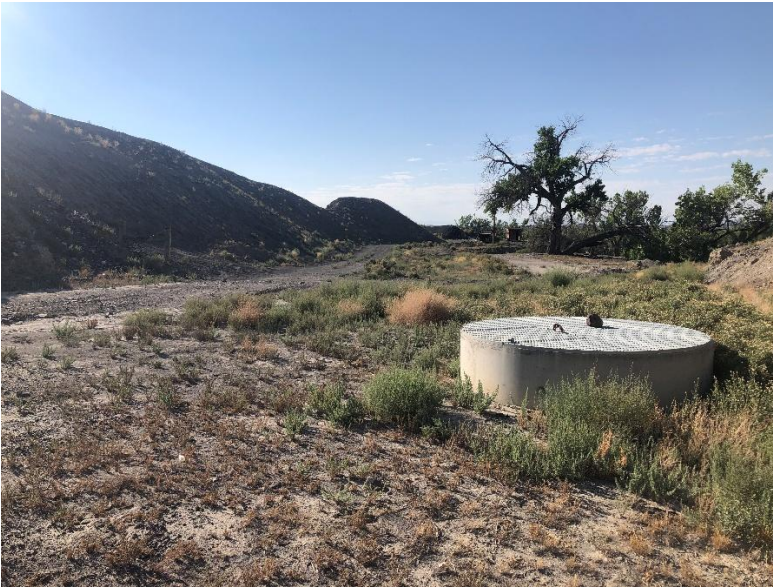
West side of affected area, with road on left, and irrigation structure for the North Delta Canal
