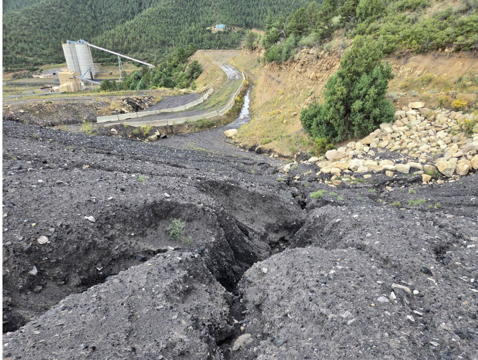
Photo 24: Looking down from the top of the RDA at the erosion gullies leading to the sediment basin by the road.
