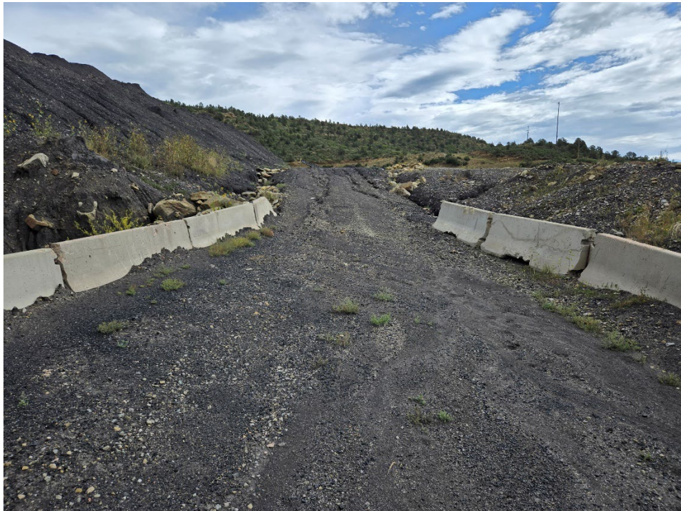
Photo 28: Looking east at the damaged check dams contributing to the sediment accumulation on both sides of the road near C81.
