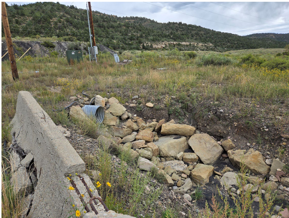
Photo 8: C65 outlet (C65 inlet also clear - not pictured)
