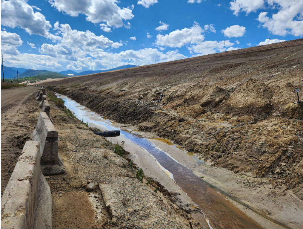
Photo 13. Horizontal drains, looking south.
