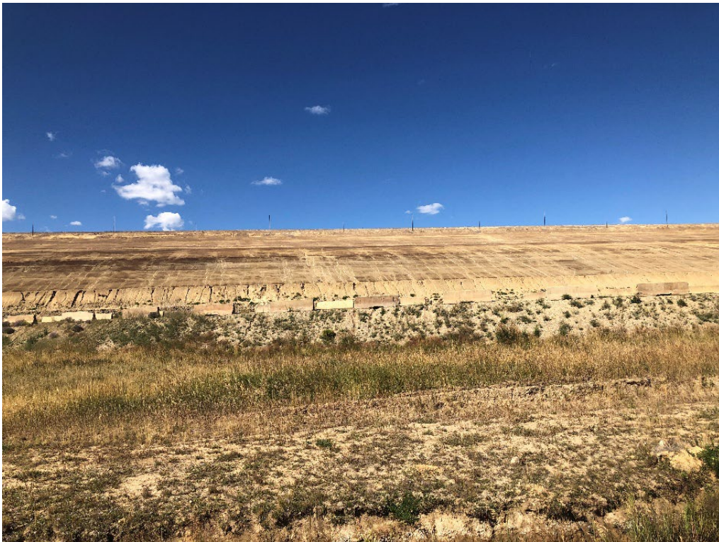
Photo 8. Small amount of erosion on face of 1-Dam, at Cell 5 area.
