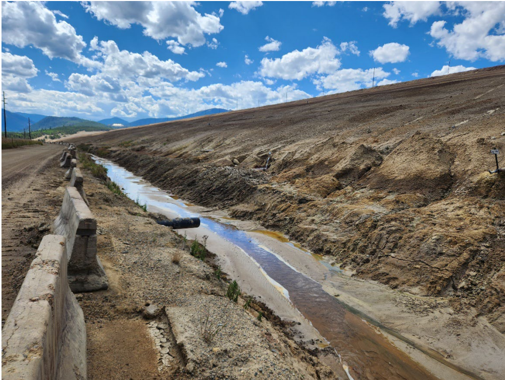
Photo 13. Horizontal drains, looking south.
