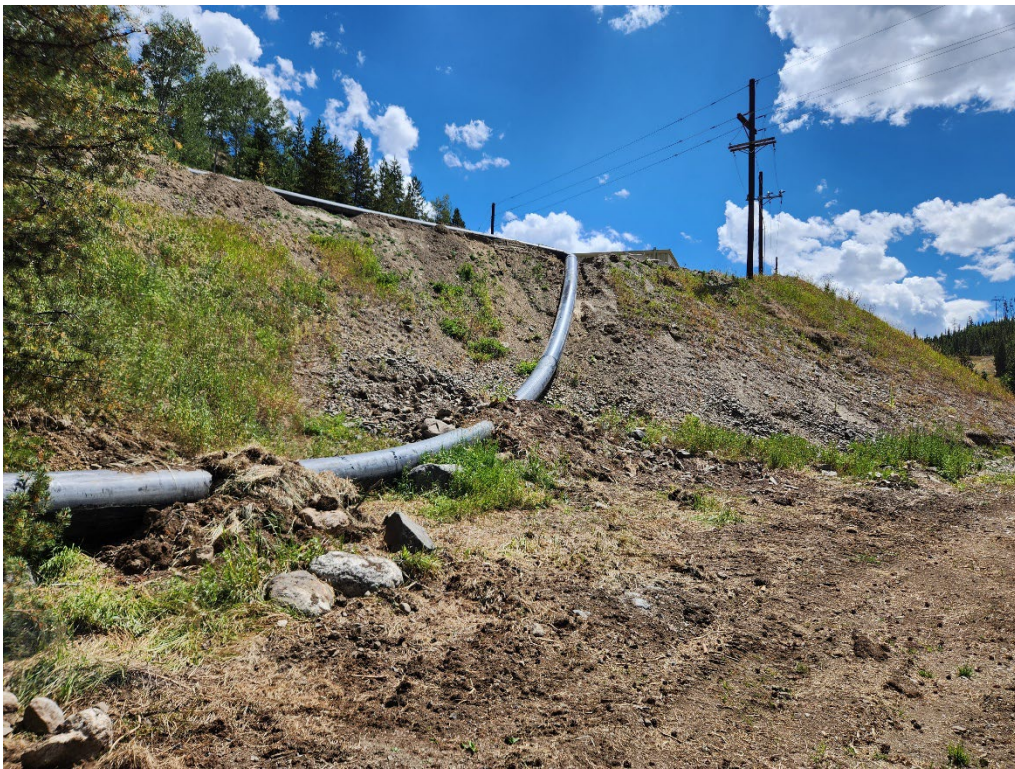
Photo 18. A 24-in leadoff pipe used to deposit tailings in the East Branch Trunk, looking north.
