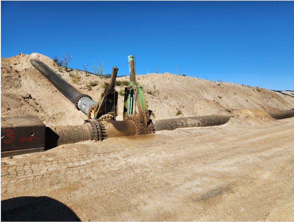
Photo 3. A spigot connection to the tailings delivery line.
