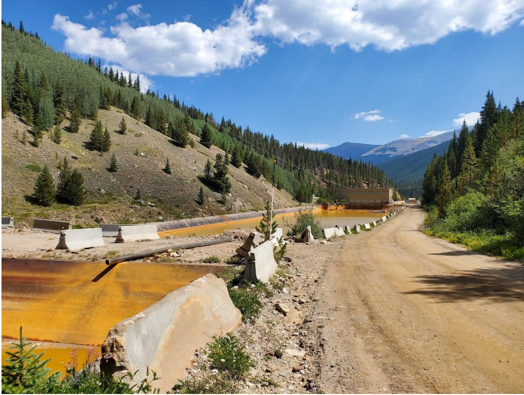
Photo 7: View to the north of 5 Dam Seepwater Collection System
