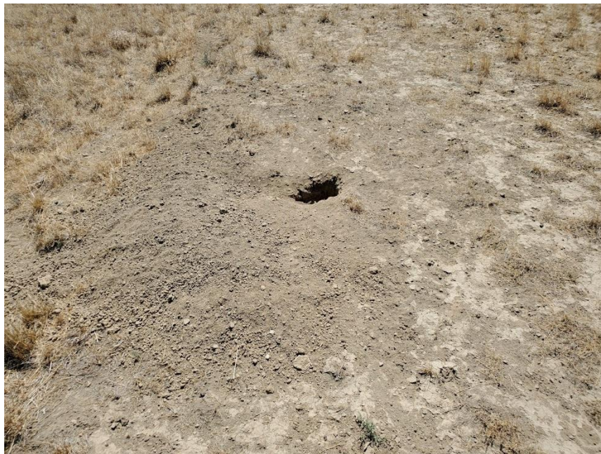
Photo 12: View to the north of animal burrow in the RP-5 embankment.
