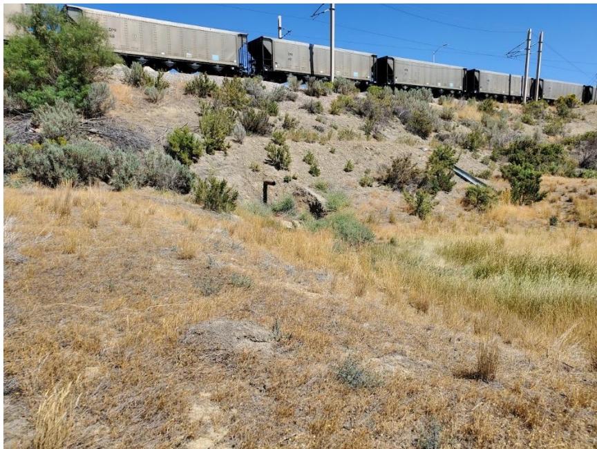
Photo 8: View to the north of the erosion scar on the rail pond. No change since last inspection.
