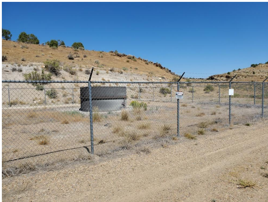
Photo 13: View to the north of animal burrow in the RP-5 embankment.
