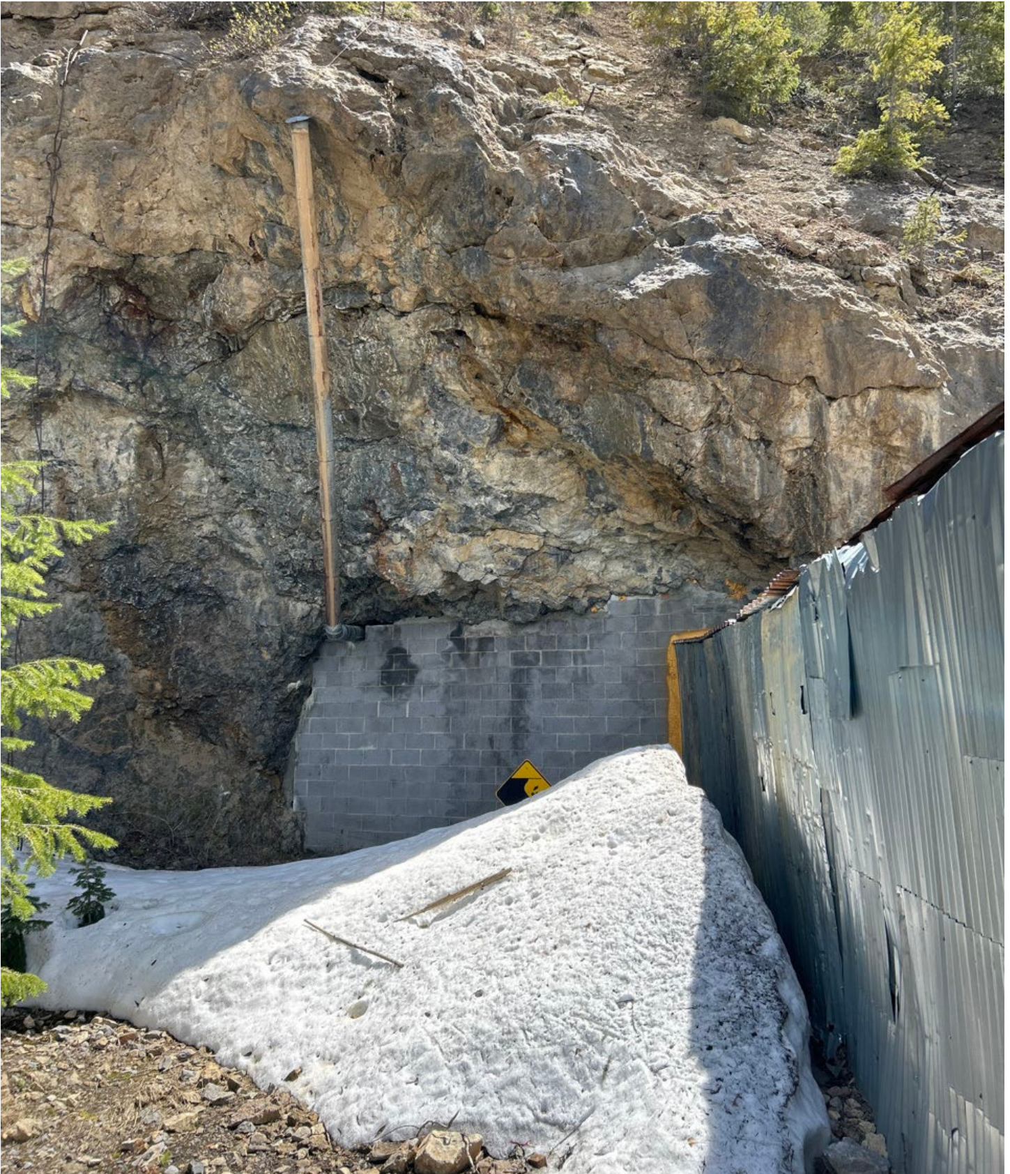
Figure 10: Blocked portion of portal entrance, adjacent to tunnel
