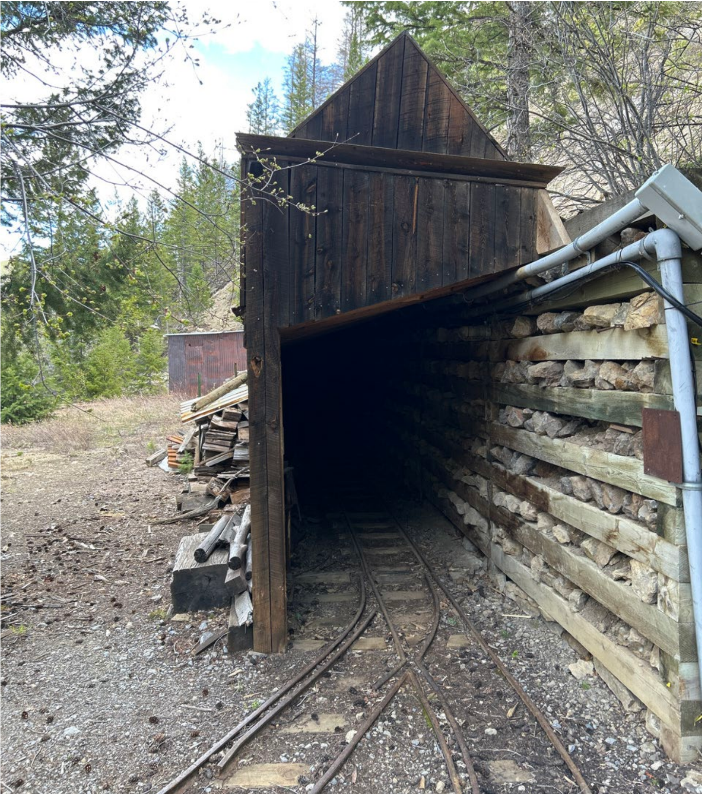
Figure 7: Covered rail between cabin and portal
