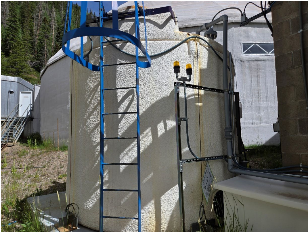
Photo 9: Insulated Sulfuric Acid tank located outside of the URAD water treatment plant.
