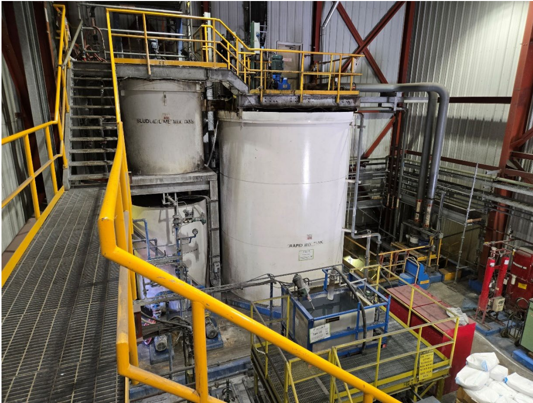
Photo 8: Floculant storage tank located within the URAD water treatment plant.
