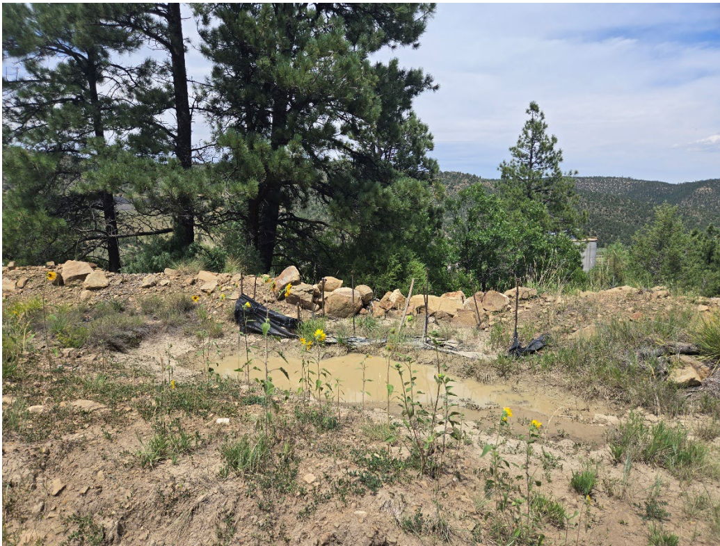
Photo 19: Looking northeast at the damaged silt fence within the S.A.E. on the southside of the permit area, near the water tanks.
