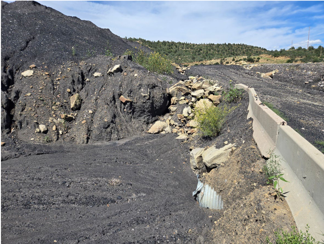
Photo 26. Looking at the damaged and eroded check dams within the ditches that lead to the inlet area for culvert C81.
