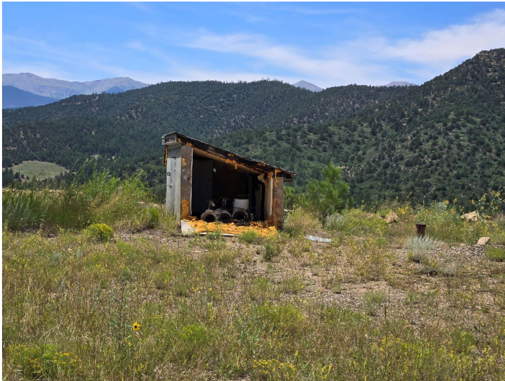
Photo 35: Damaged water pump/valve cover structure.
