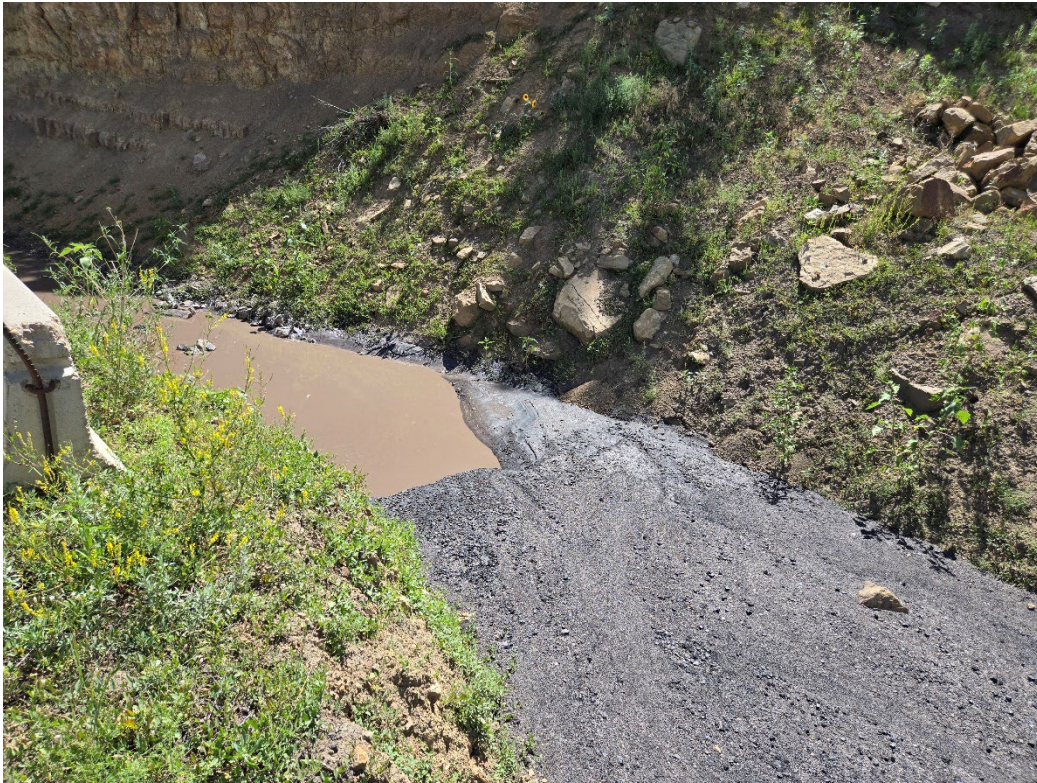
Photo 23: Looking at sediment accumulation and water held in Ditch D56 at the time of the inspection.
