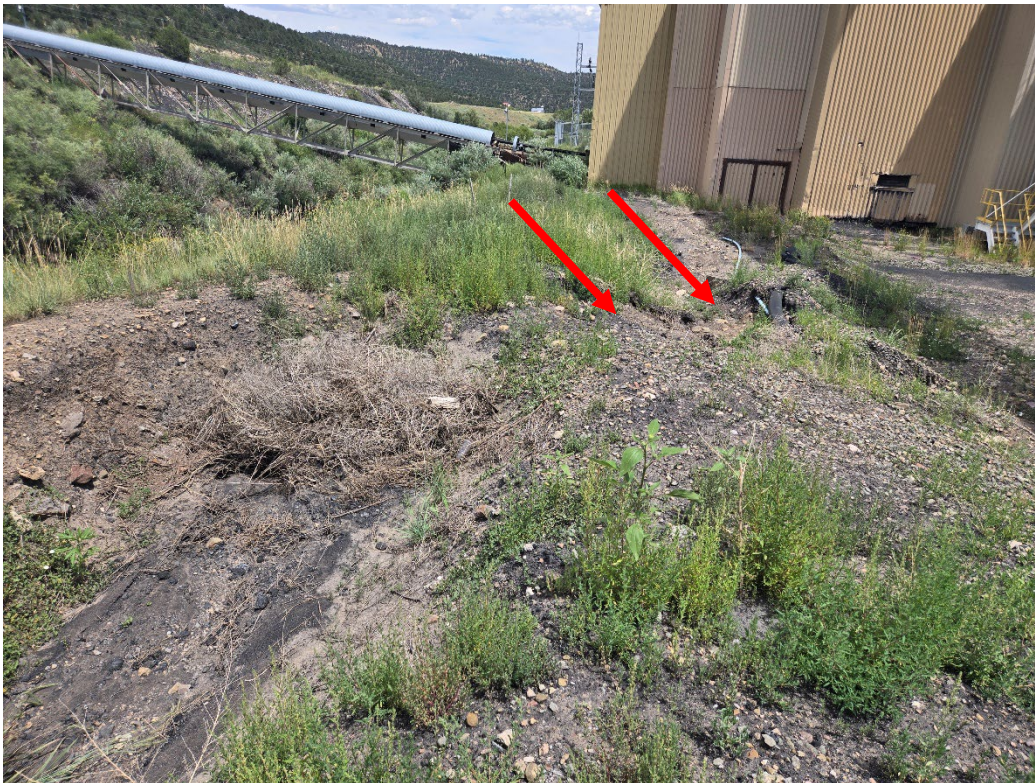
Photo 20: Tumbleweeds and other debris block the inlet for culvert C64. The arrow points to where water had overflowed in the ditch and discharged into the Raw Coal Storage area.
