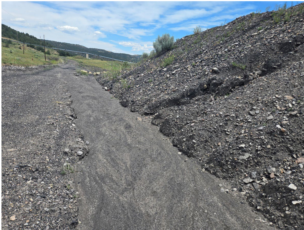
Photo 7: Sediment in D12 along the north side of DWDA #2.
