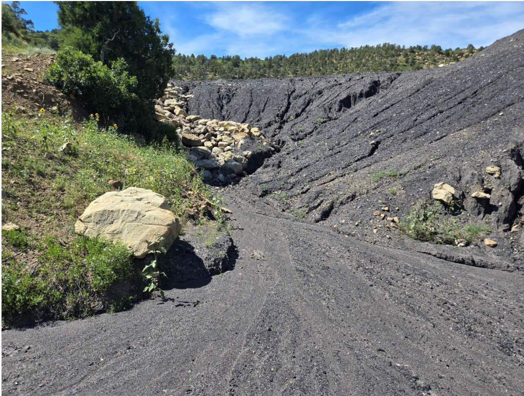
Photo 27: Looking north at the excessive erosion on the west side of the RDA slopes.
