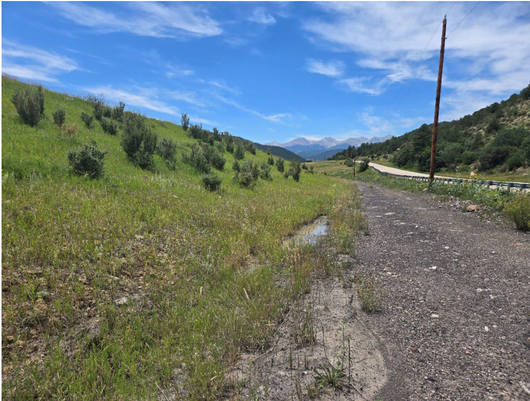
Photo 3: Looking west at an area where sediment from ditch D2 has begun to erode the road leading to Pond 004a.
