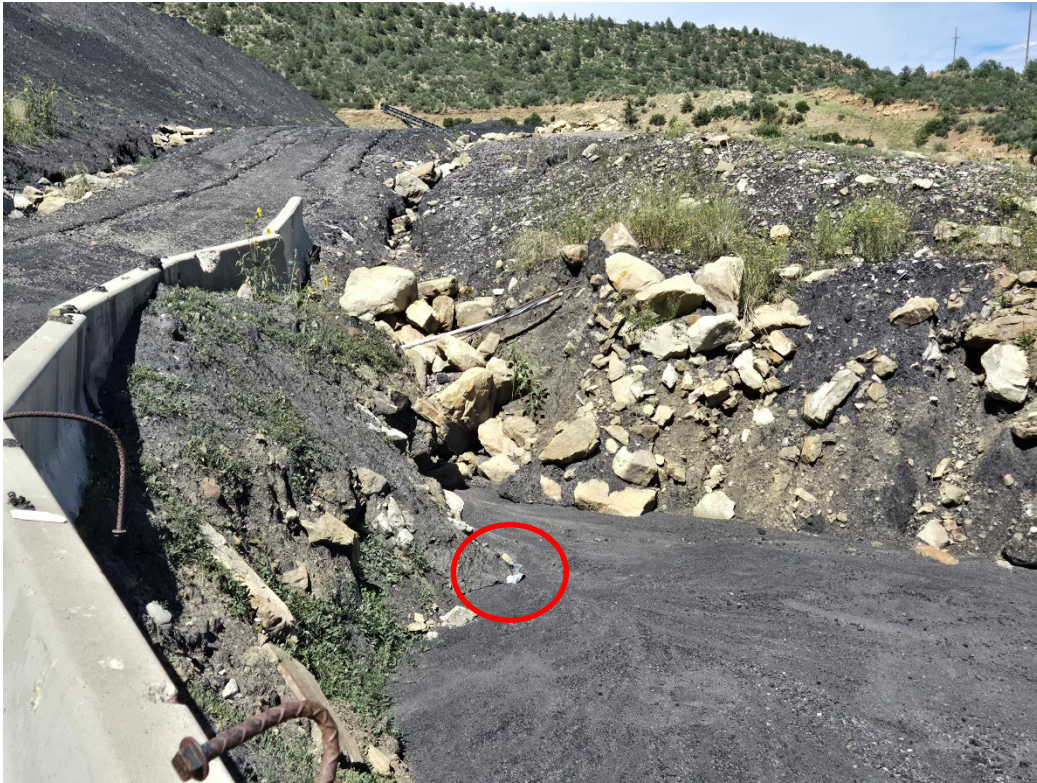
Photo 25: Looking at the damaged and eroded check dams within the ditches that lead to the outlet area for C81. The red circle shows the very top of the now buried C81.
