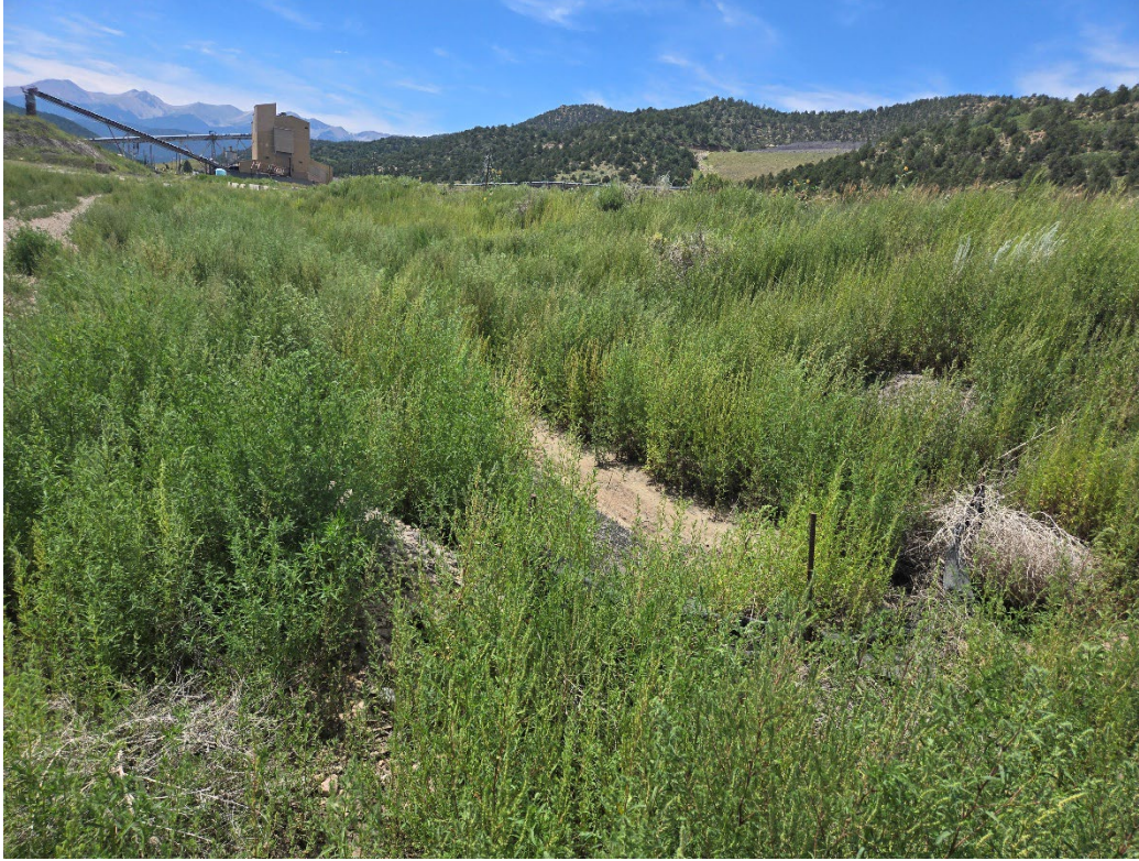
Photo 18: Looking west along the damaged silt fences on the north side of the road in the S.A.E. on the south side of Pond 007a.
