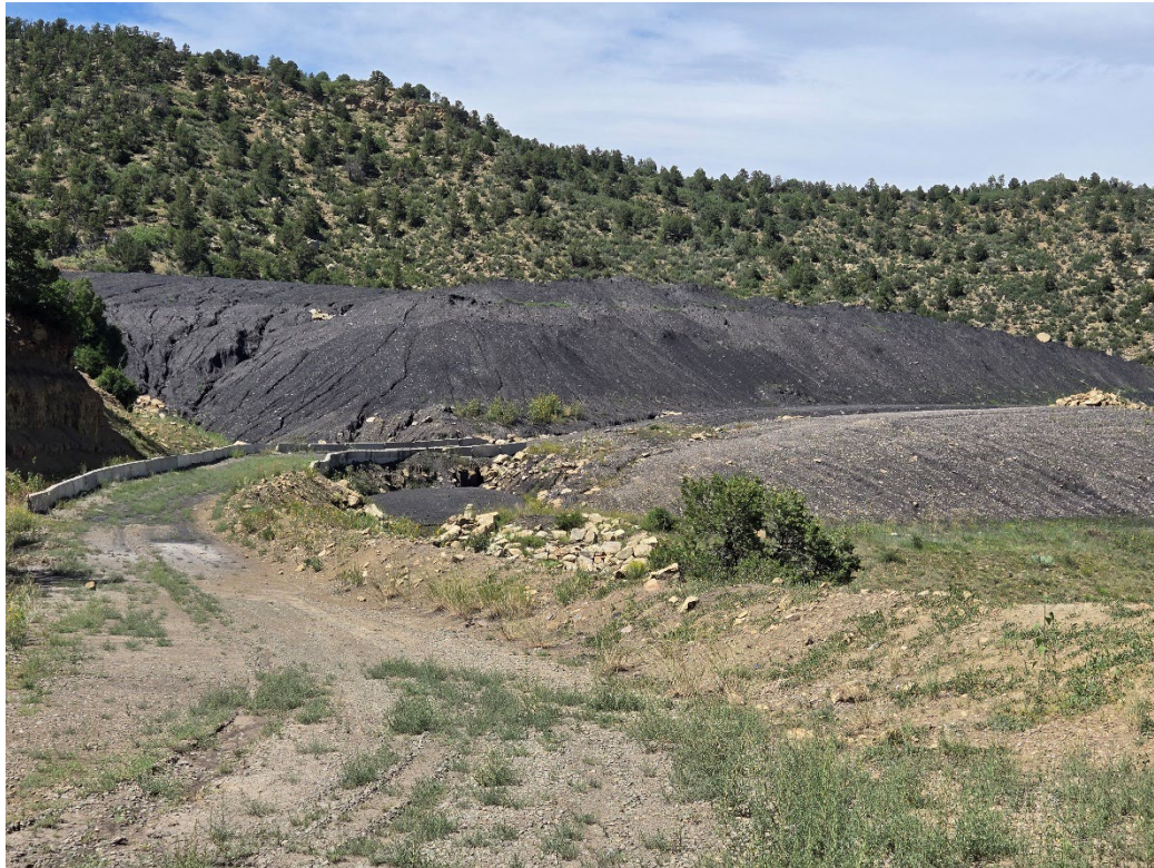
Photo 22: Looking north at the significant erosion occurring on the west side of the unclaimed RDA areas that lead to C81.
