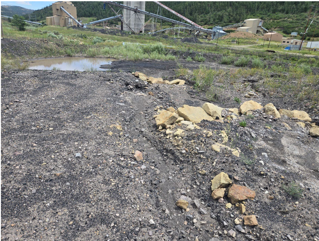
Photo 8: Check dam full of sediment at the east end of ditch D12. The sediment has overflowed and cut around the check dams, but is still being deposited in the sediment basin.
