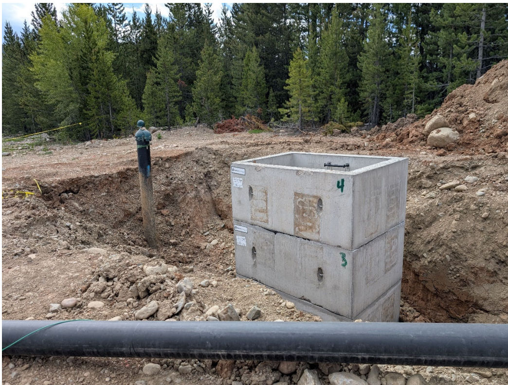
Photo 4: Looking at extraction well MLEX 7 and vault installed on the south end of the gravel pit.
