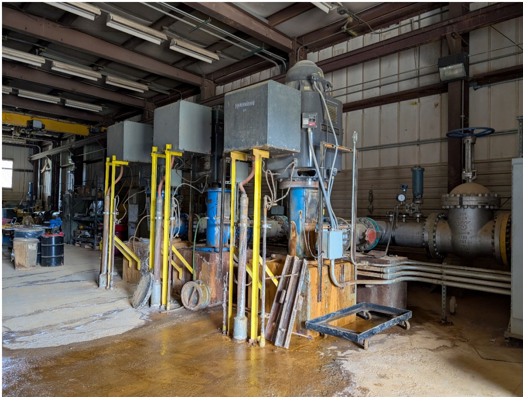
Photo 16: Looking at the pumps inside the Ute Park Pump Station.
