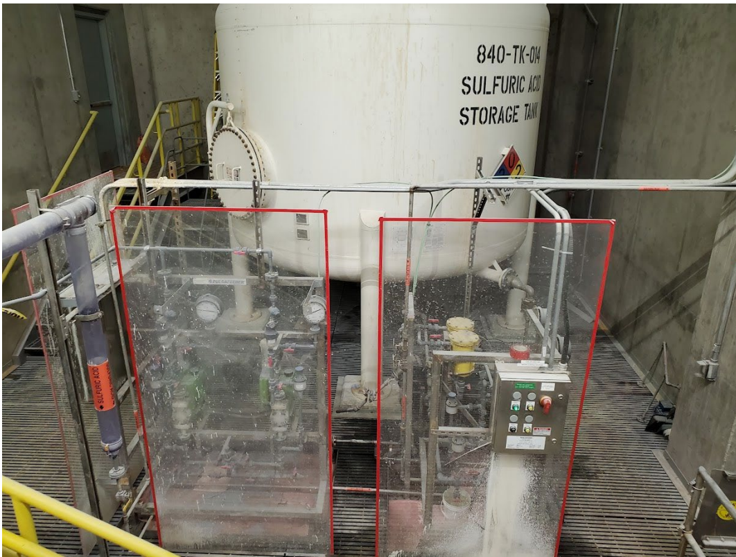
Photo 8: View to the west of sulfuric acid storage in the PDWTP.
