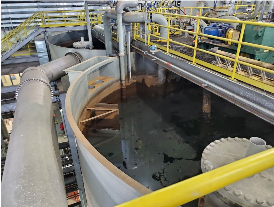
Photo 7: View to the east of the reactor tank in PDWTP.
