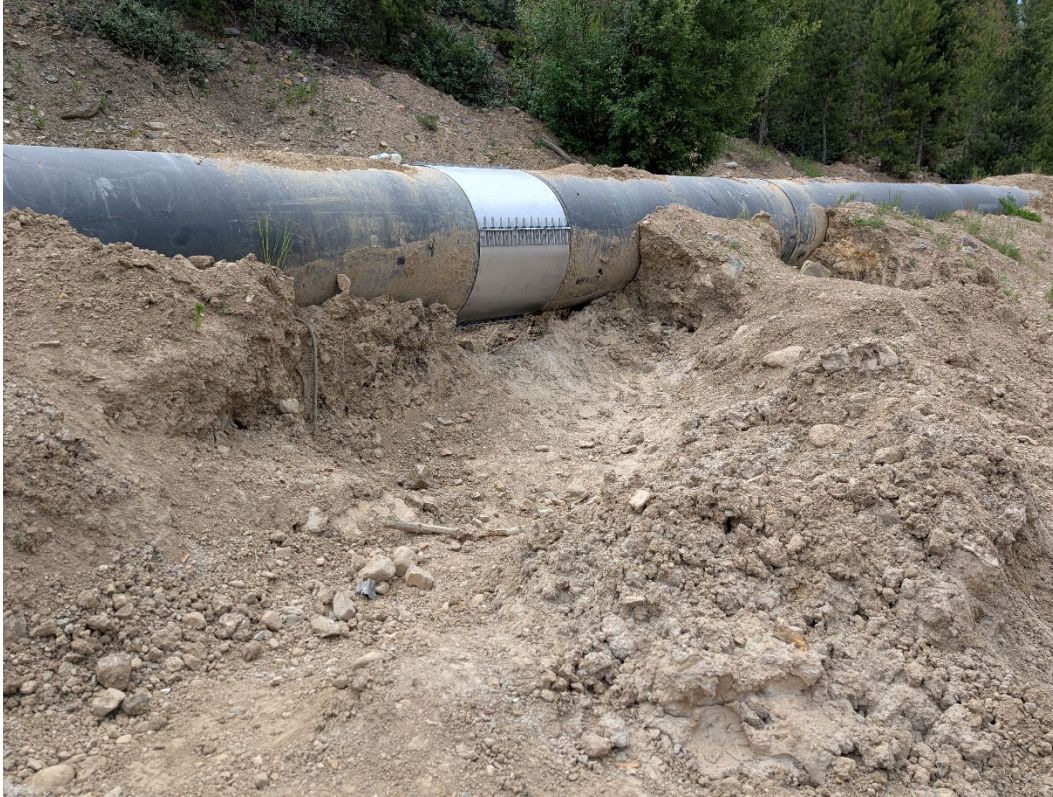
Photo 3: Looking at a temporary metal band installed on the TDL where a leak was observed.
