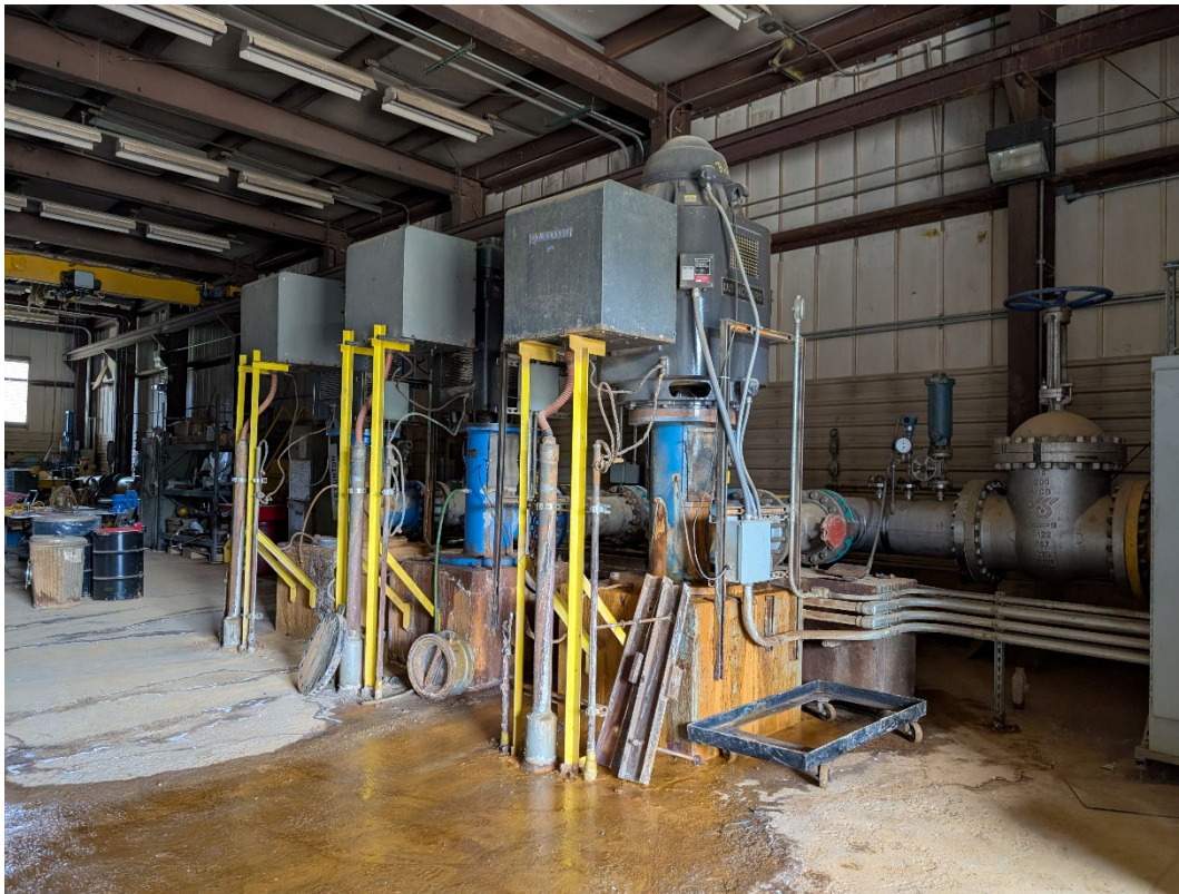
Photo 16: Looking at the pumps inside the Ute Park Pump Station.
