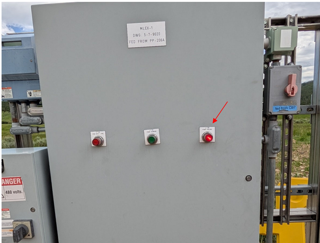
Photo 8: Inspection of extraction well MLEX-01. The well was not operating during the inspection. Red light indicates well is off.
