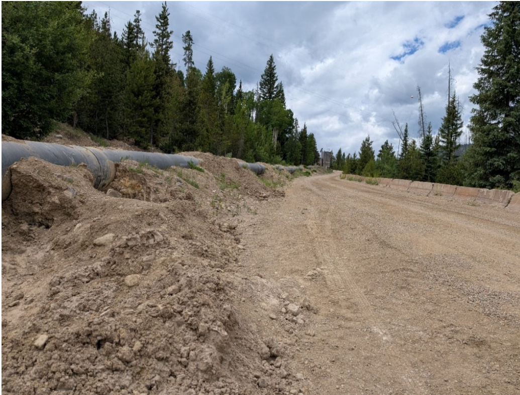
Photo 1: Looking at the TDL in a steep section above 3-Dam, below the No. 1 Cutout.
