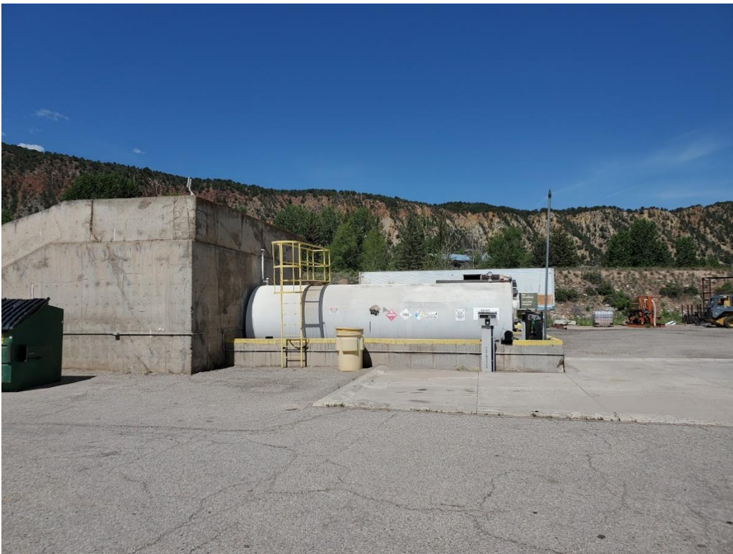
Photo 2: View to the west of fuel storage on site.
