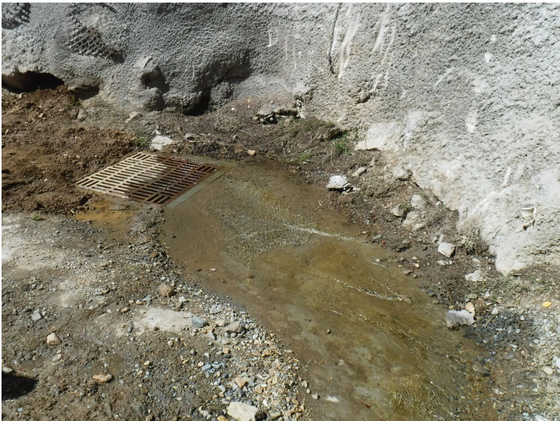
Photo 2: Idaho Tunnel effluent discharge directed to grated drop structure to enter pipeline
