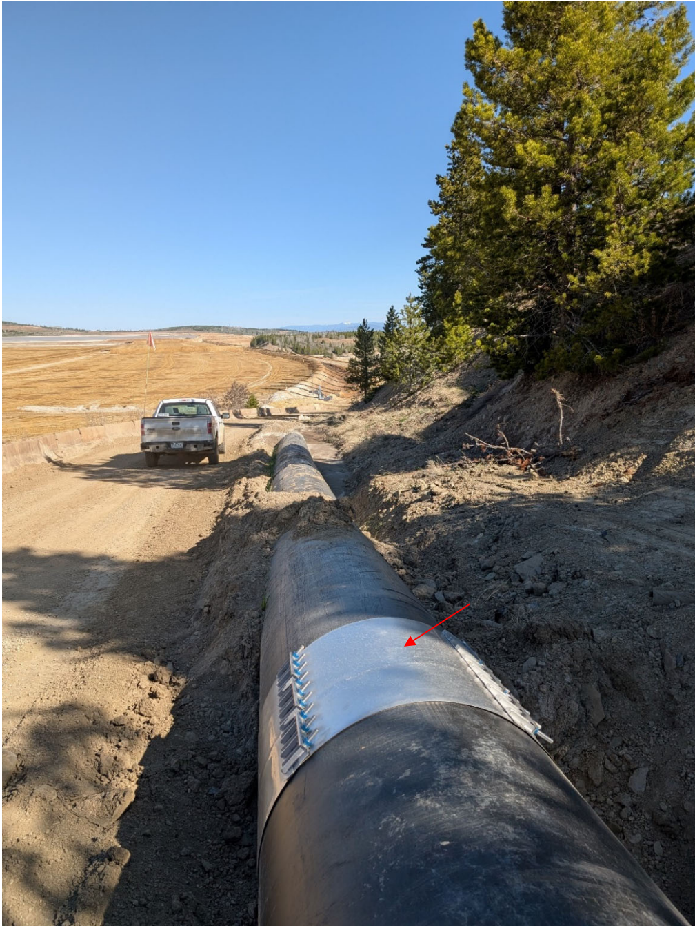
Photo 2: View looking northeast at the Tailings Delivery line, adjacent access road, and beginning of 3-Dam. The banded section is where the leak occurred (red arrow). Tailings flowed along the access road and the spill was contained in this area.
