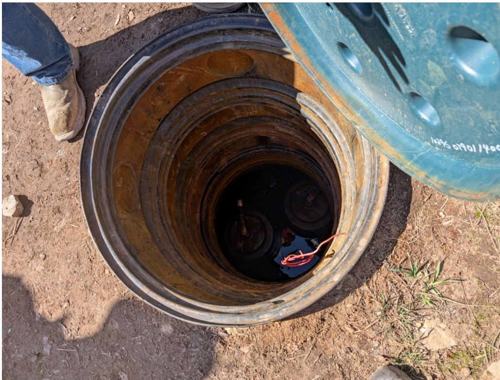
Photo 8: Looking down at siphon valves within a seep water vault.
