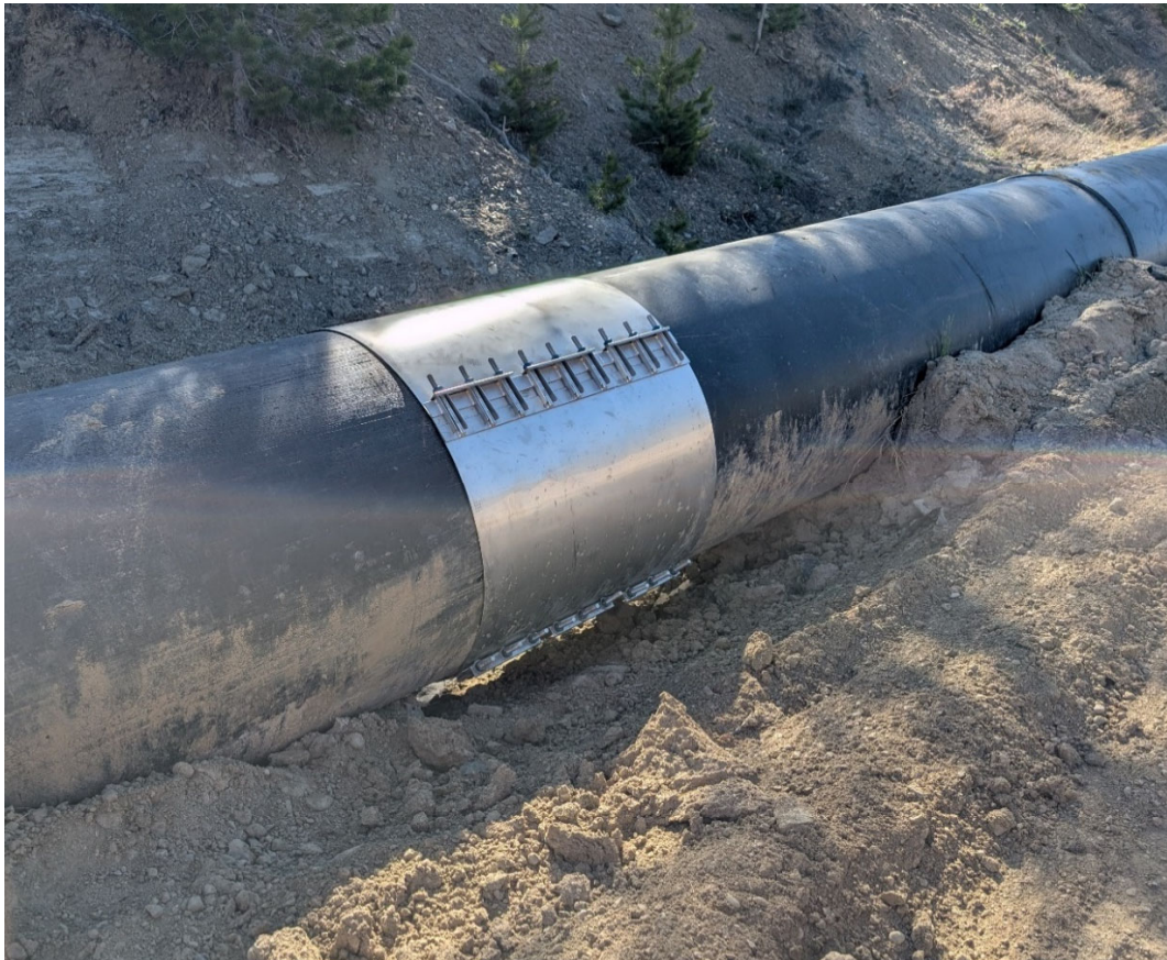
Photo 1: Looking at a section of the HDPE tailings delivery line where the leak occurred. A metal banded clamp was used to repair the pipe.
