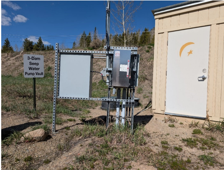
Photo 11: Control station and pump house for the seepwater collection system below 3-Dam.
