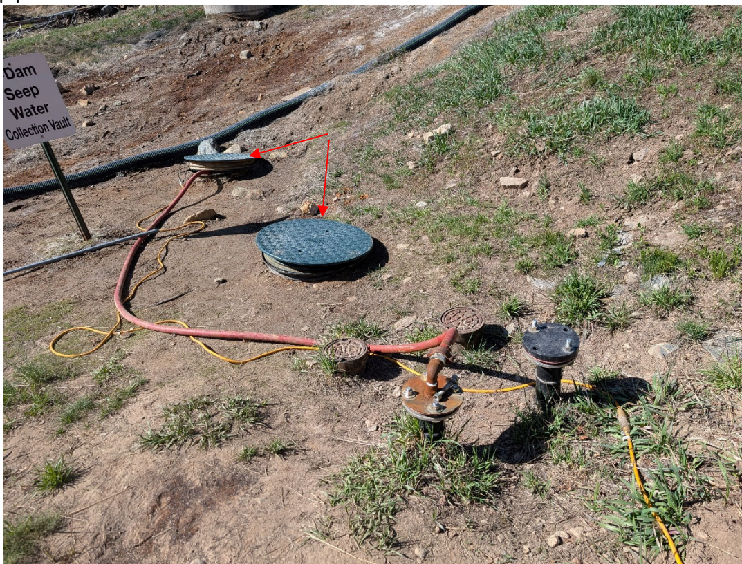
Photo 6: 3-Dam seepwater collection vault covers.
