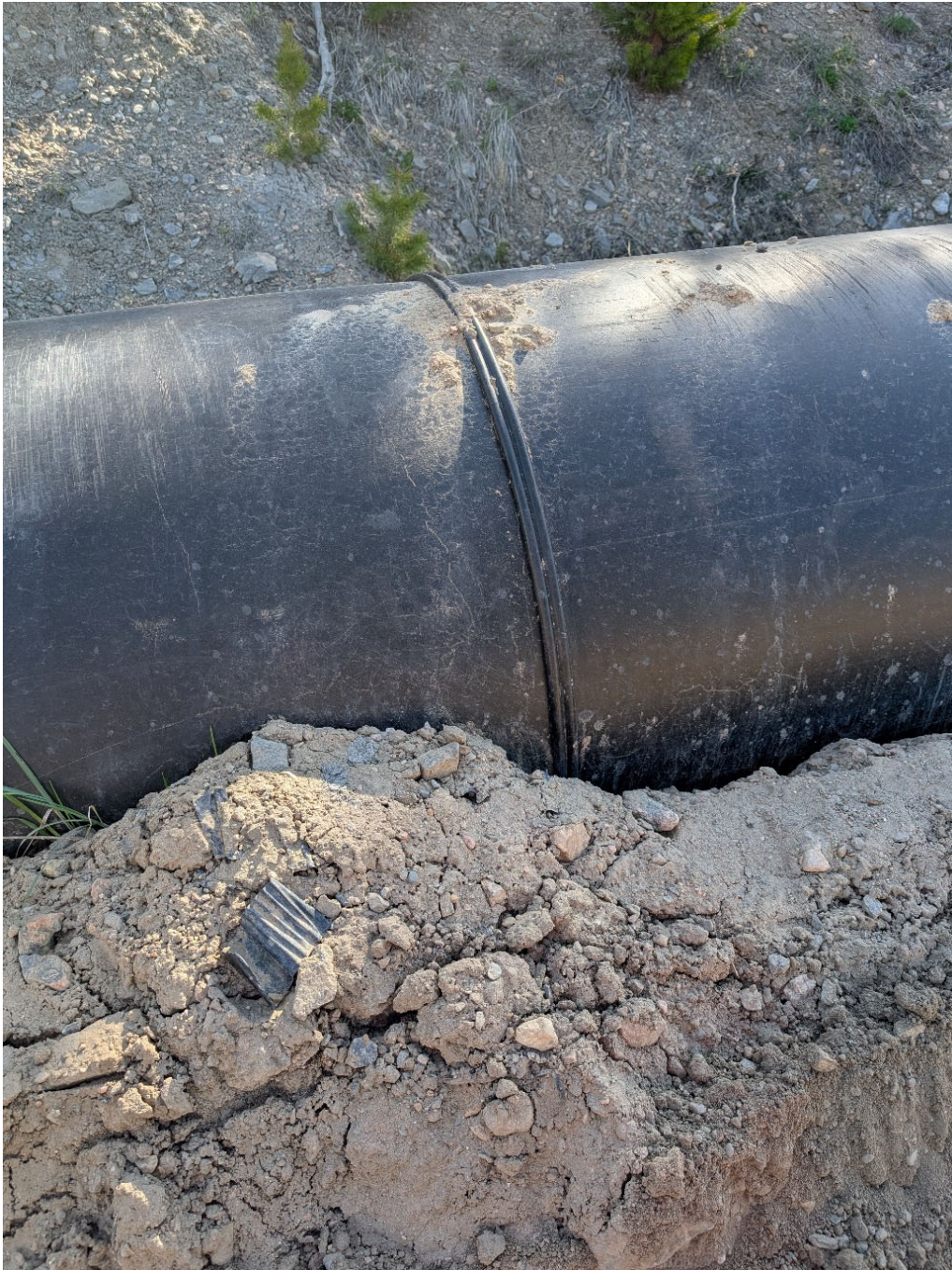
Photo 4: Connecting joint along the HDPE tailings line. Over time, the pipe tends to scour at these joints, especially in steeper sections.
