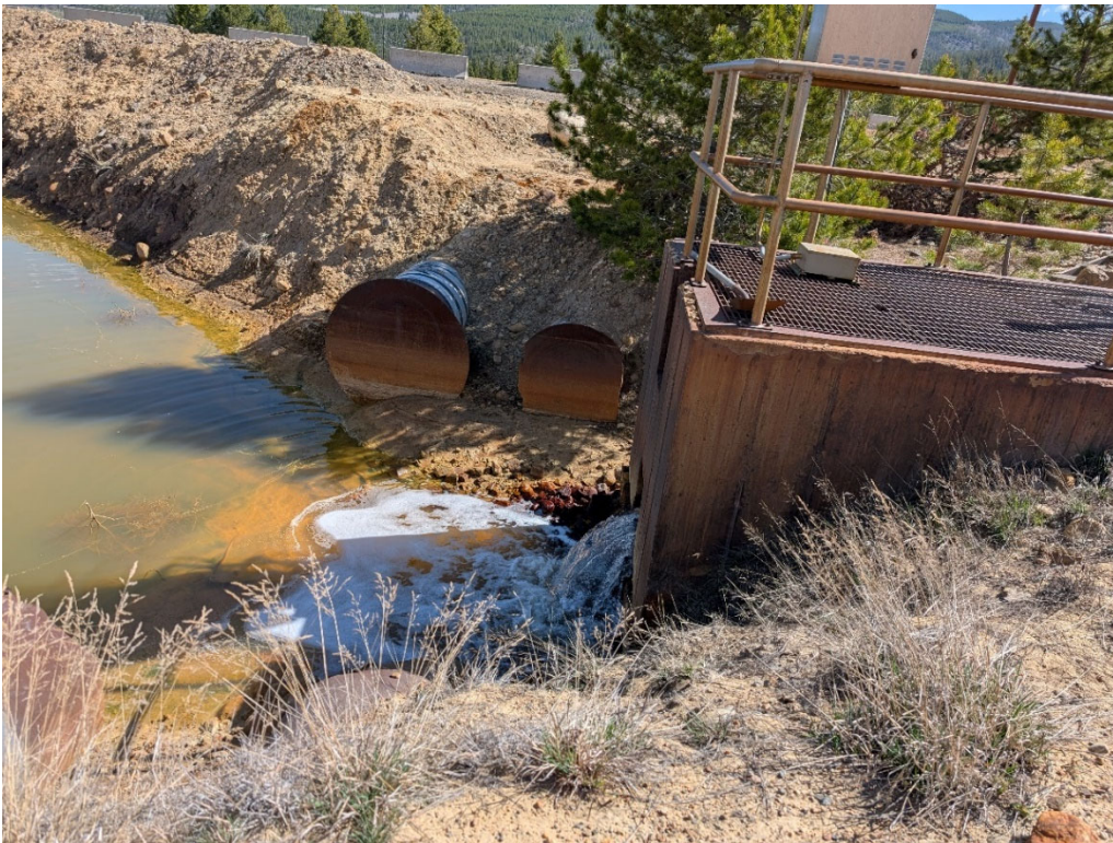
Photo 14: Looking at the outlet for the main seepwater return pipeline located at the base of 1-Dam near the Ute Park Pump station.
