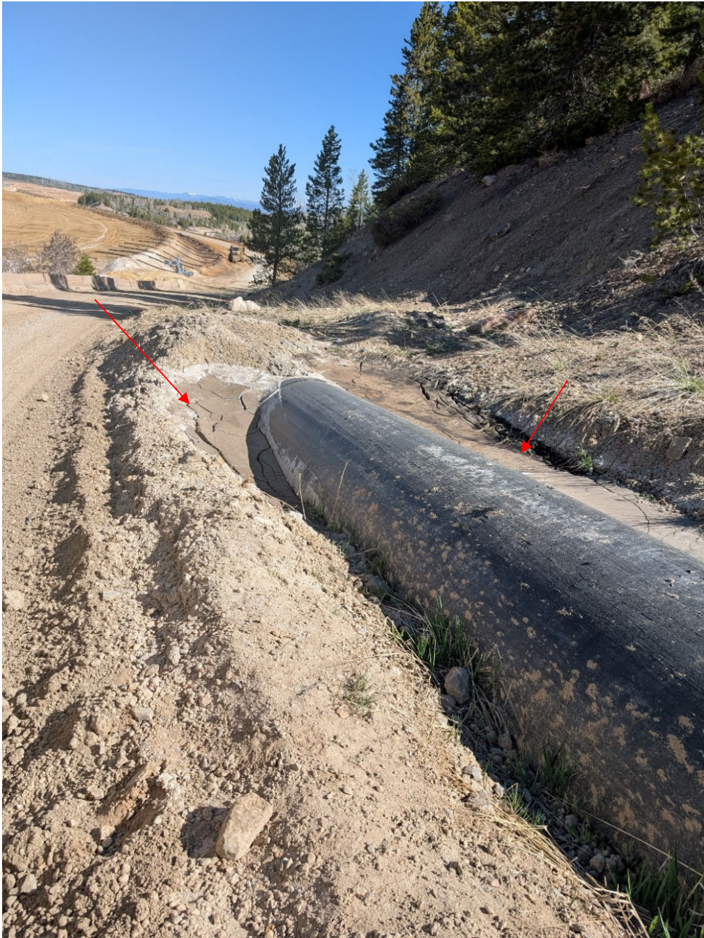
Photo 3: Looking at the area where the spilled tailings slurry accumulated when it leaked out of the HDPE pipe.
