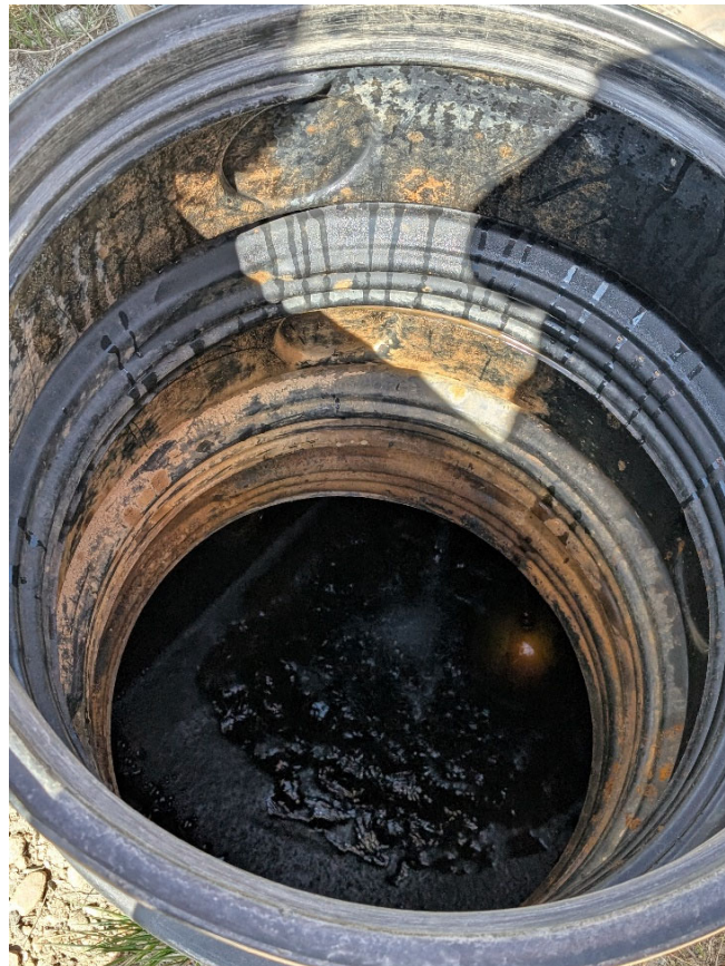
Photo 12: Looking down into the 3-Dam seepwater pump vault. Water is pumped to the main return pipeline.
