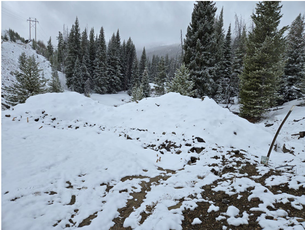
OF-M04 (Photo 12) The BMPs of this outfall location consist of wattles in front of a rock check dam leading to a rip-rap outfall. These structures were covered in snow at the time of inspection. The sign had fallen off the post.
