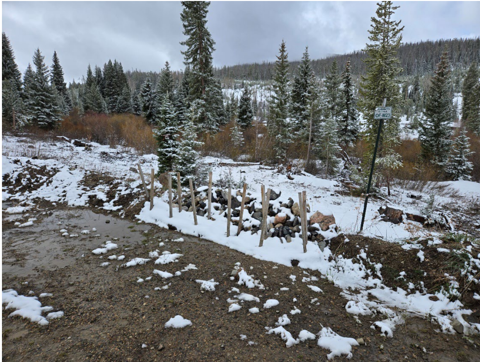
OF-M23 (Photo 16) - The BMPs of this outfall location consist of wattles in front of a rock check dam leading to a rip-rap outfall. This outfall has a small drainage collection area and was not holding a lot of water or excess sediment at the time of the inspection. Some water appeared to be pooling on the sides of the wattles and rock check dam, but the structure appears to be working well.
