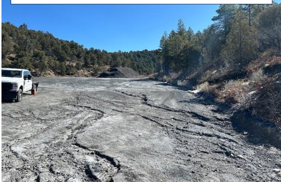
Photo 18: The top of the URDA with rills observed draining into the west drainage (Rach 10).
