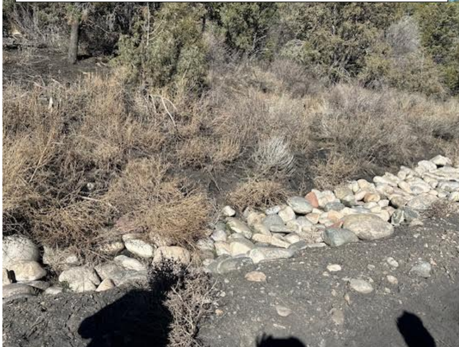
Photo 4: The hillside above the west clearwater ditch referenced in Maintenance Item #3.
