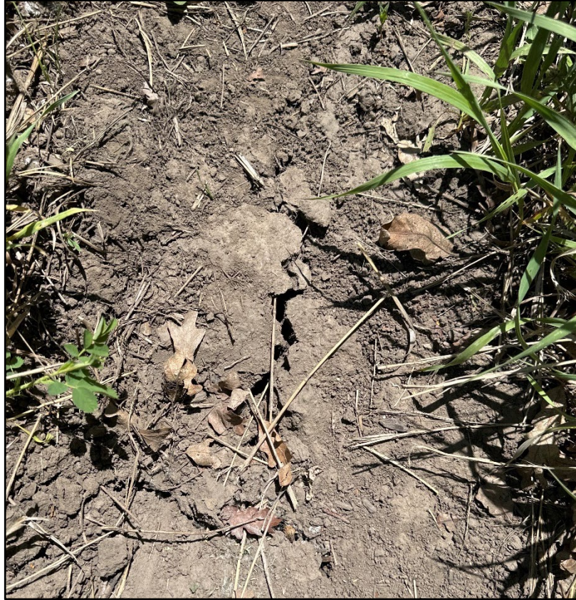
Figure 1: Small subsidence crack on trail along Horse Gulch overlying Longwall Panel E12.
