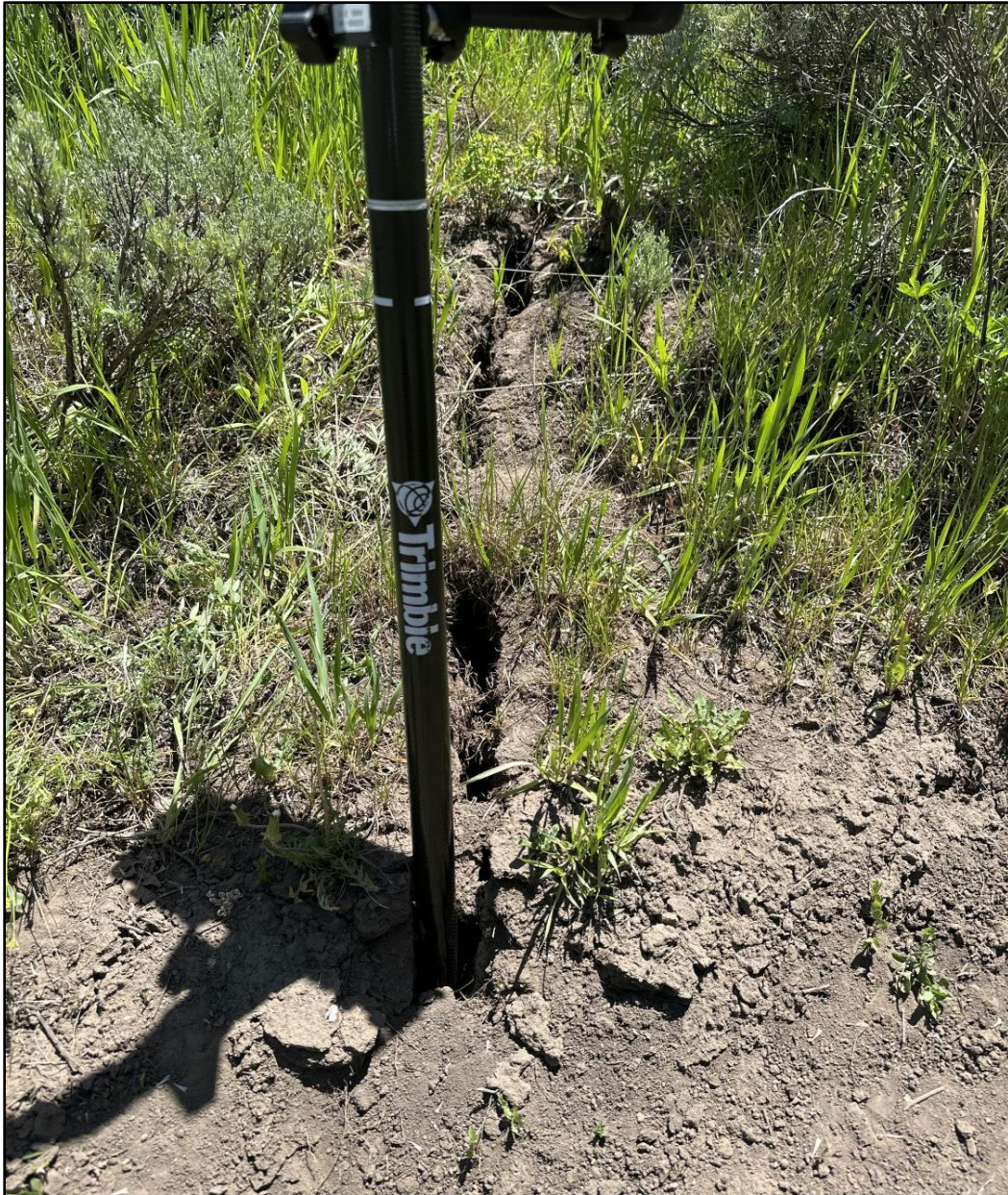
Figure 4: New crack observed over Longwall Panel E15 during spring 2024 site visit
