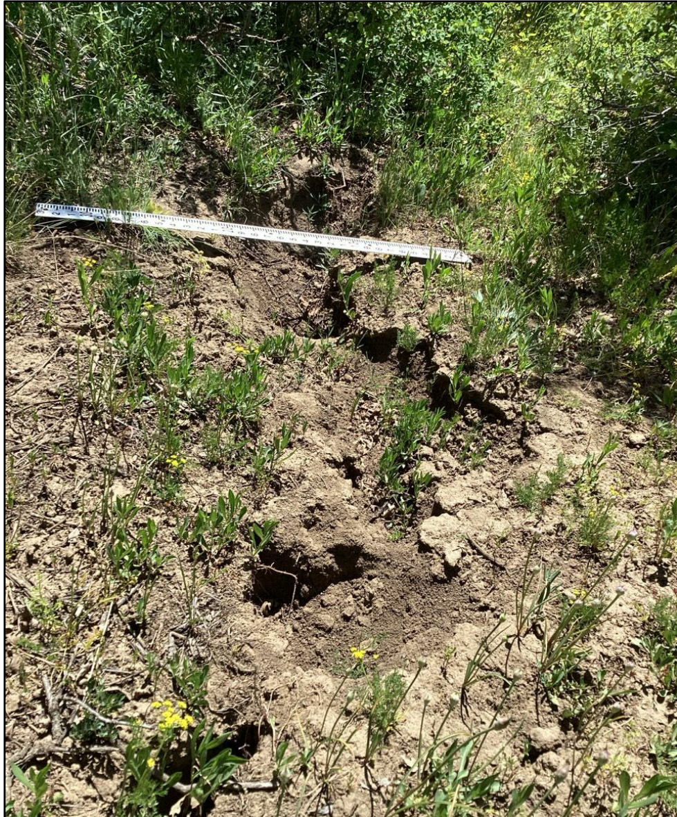
Figure 3: One of the largest of the cracks at Location 2, south of the across road on Traverse C-C' during spring 2024 visit showing continued healing.
