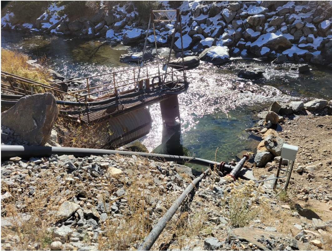
Photo 5: Pipeline and inlet on Clear Creek adjacent to the mine office.
