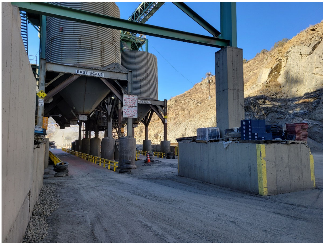
Photo 2: Looking at the newly installed truck scale in the loading area.
