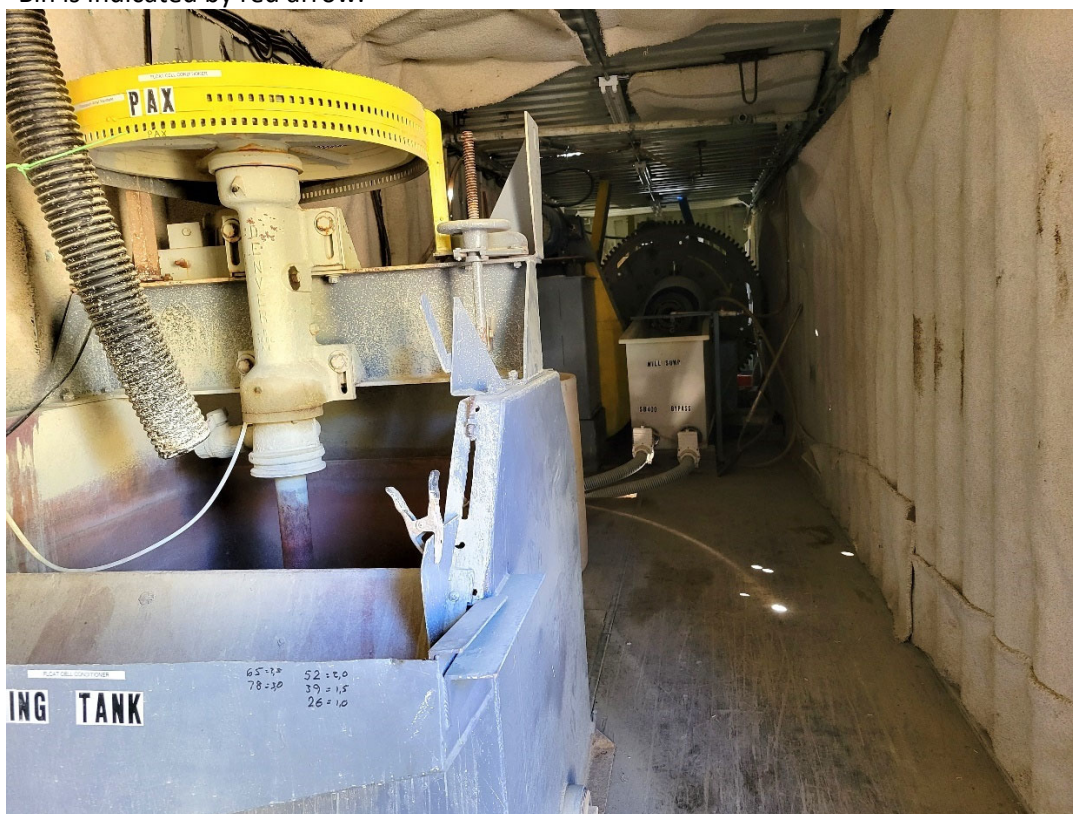
Photo 4: Inside view of the Ball Mill Trailer.
