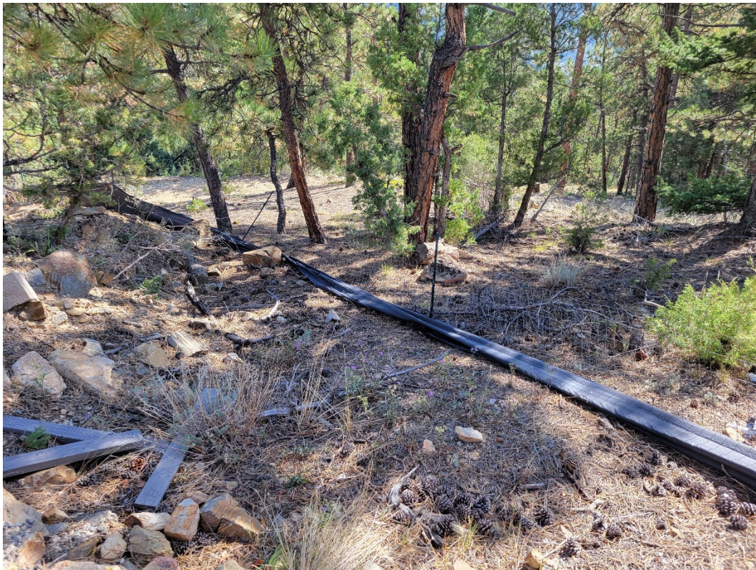
Photo 8: View of non functioning silt fence on the east side of the permit area.
