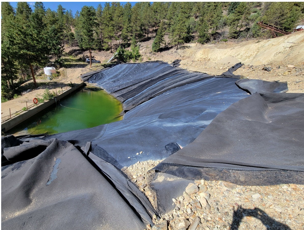
Photo 17: Looking at weathered composite liner. Top layer is blow off and laying above the Tailings Storage Impoundment.
