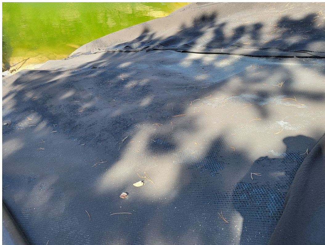
Photo 16: Closeup view of the weathered liner in the Tailings Storage Impoundment.
