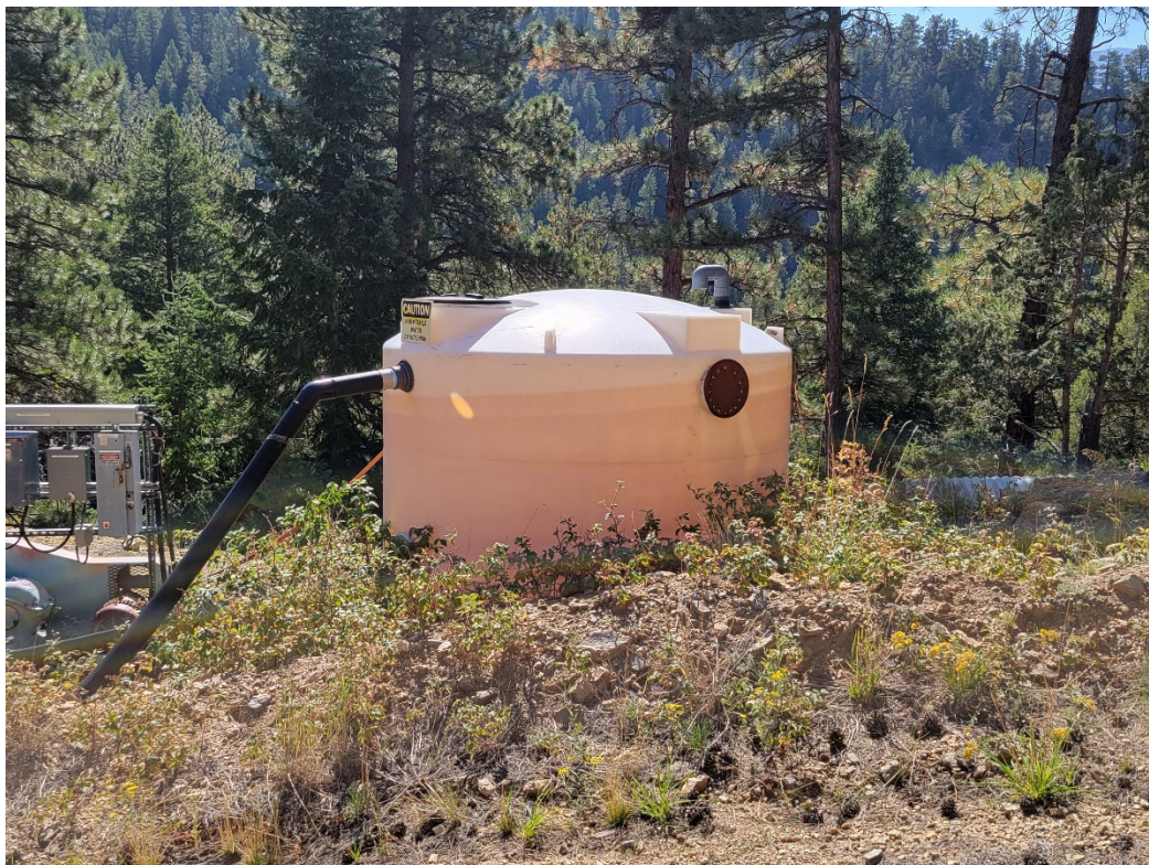
Photo 20: Process water storage tank adjacent to the Tailings Impoundment.
