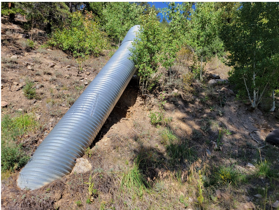
Photo 19: Stormwater diversion pipeline on the west side of the Tailings Impoundment Area.
