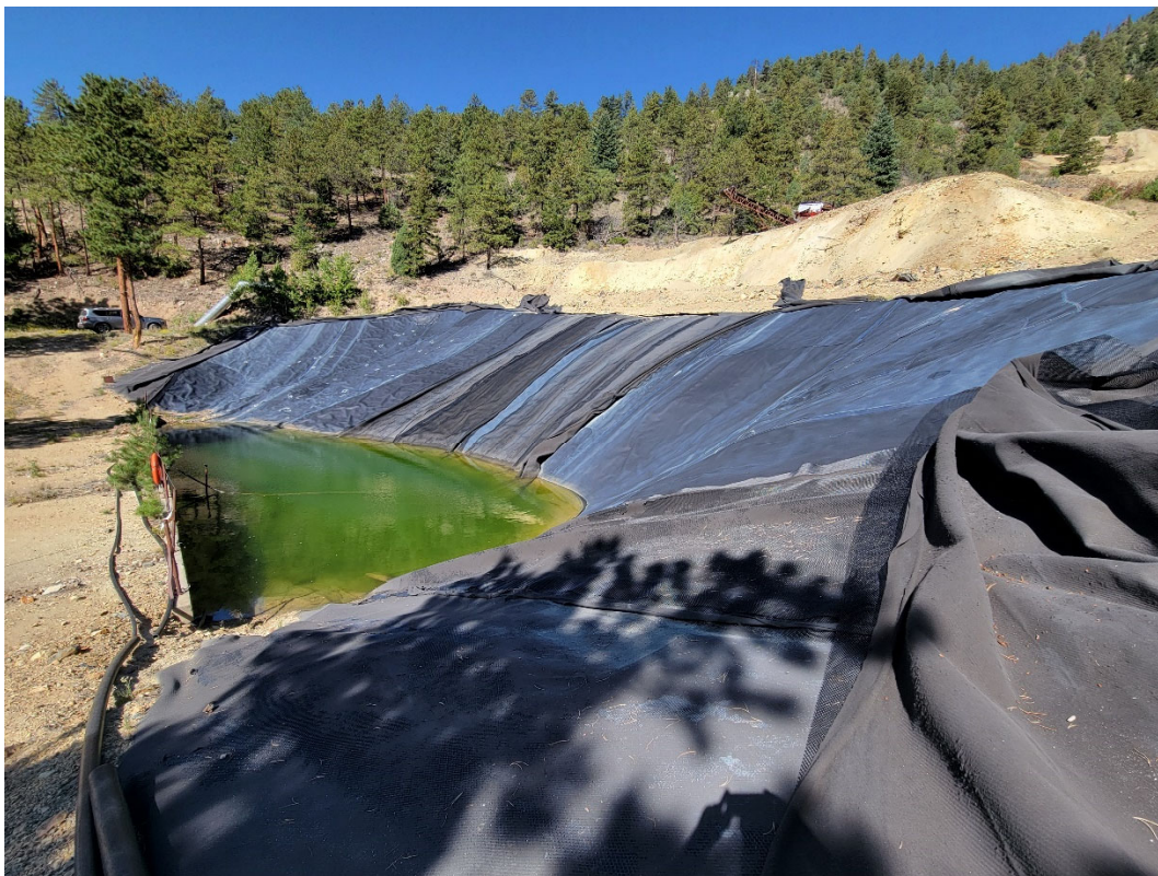
Photo 15: View of poorly maintained liner system within the Tailings Storage Impoundment.
