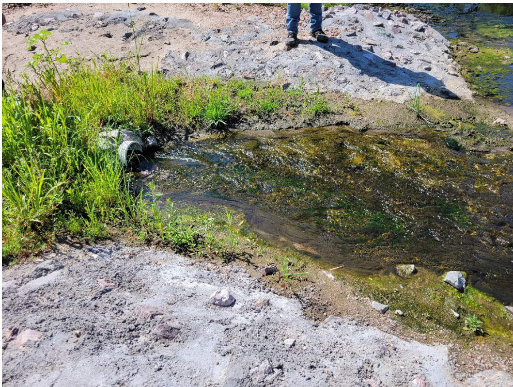
Photo 9: Looking at the outlet for the groundwater drain in the South Platte River.
