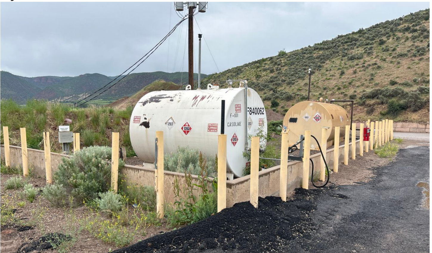
Figure 13: Fuel tanks. Point 312
