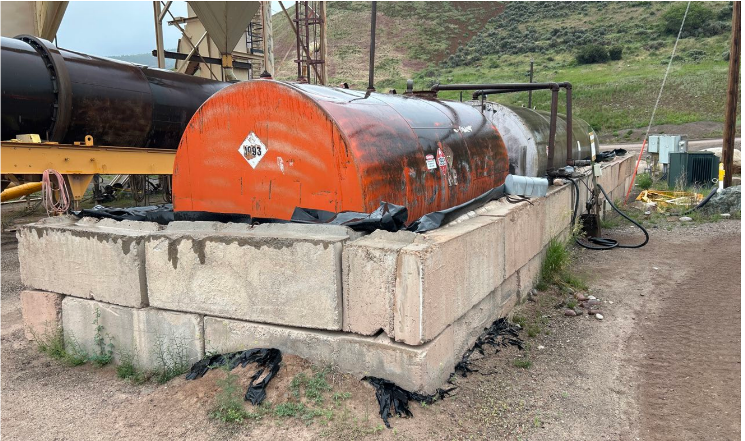
Figure 12: Fuel tanks. Point 311
