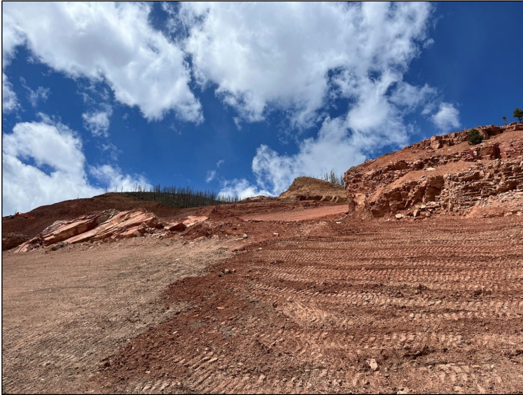
Photo 9: View west from beneath the tension crack area, no mounding or bulging of material in this area was observed.
