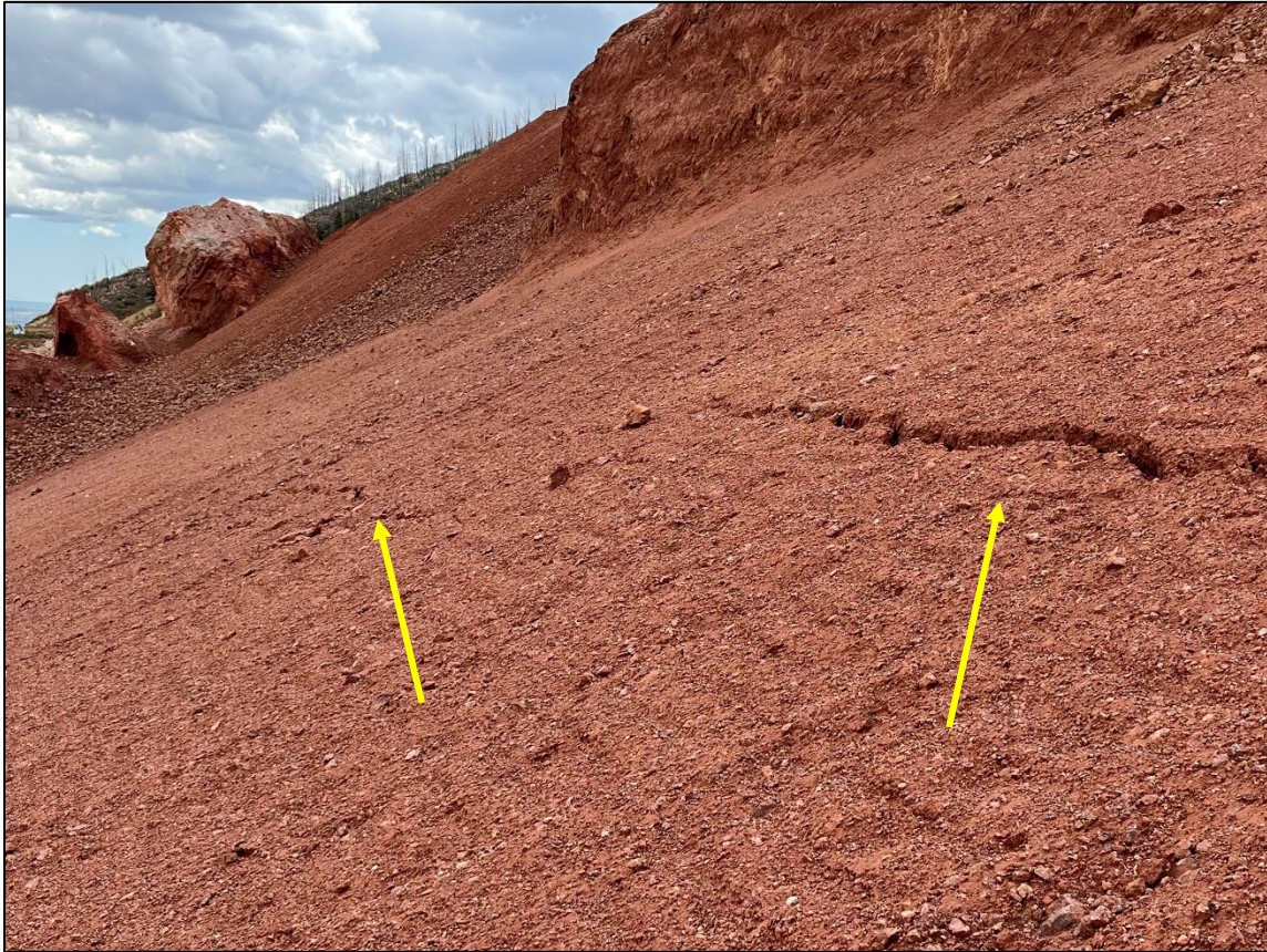
Photo 5: View south of the two cracks noted on the upper fill slope.
