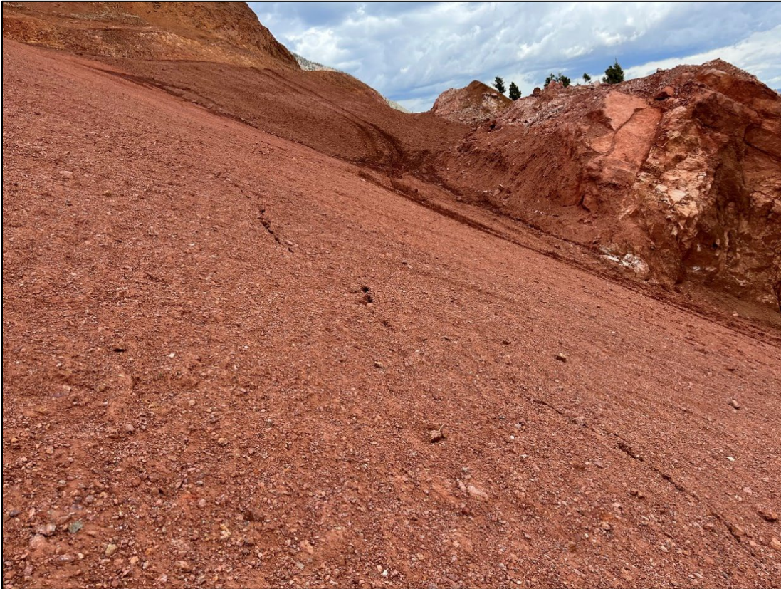
Photo 7: View facing north showing a small, third crack feature on the upper fill slope, located just above the Kiewit Cliffs feature.
