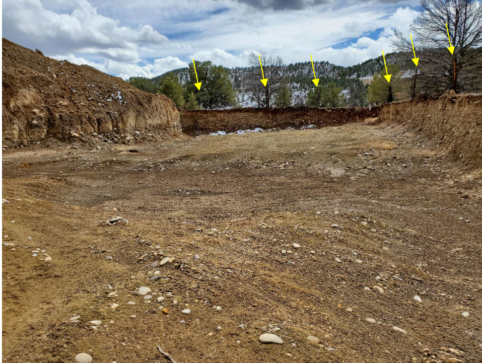
Photo 7: Looking south at the southern-west corner of Area 1. The arrows point to fence posts along the top of the highwalls.
