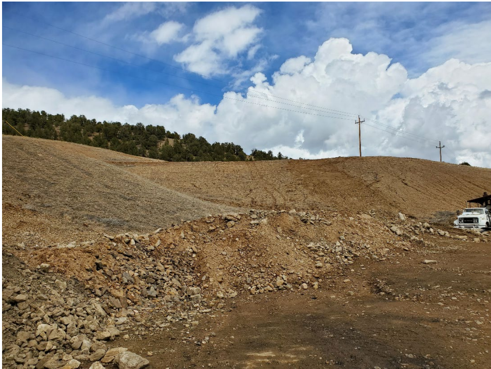
Photo 24: Looking north-east along some reclaimed slopes in Area 1. Some rilling is seen along the slopes that will need to be addressed.
