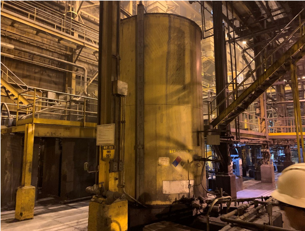
Photo 5 – Main Tergitol NP-9/N9N storage tank.
