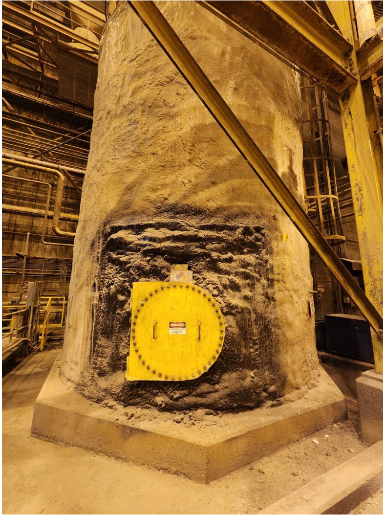
Photo 8 – Nokes storage tank.
