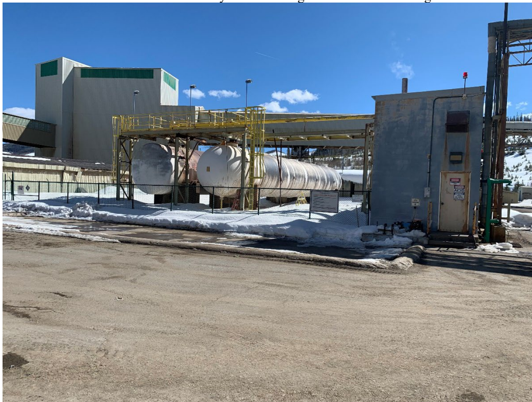
Photo 2 – HCL storage tanks. The left tank (north) is not being utilized
