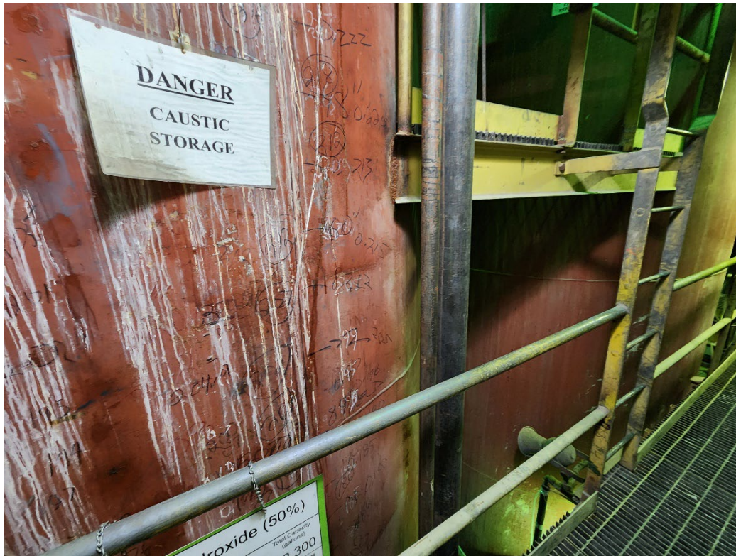
Photo 1 – Sodium Hydroxide storage in the Nokes building.
