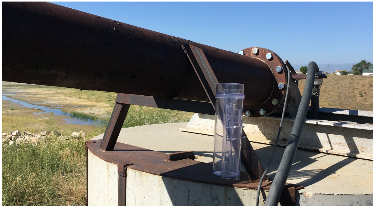
Figure 9- Rain gauge installed at wet well.
