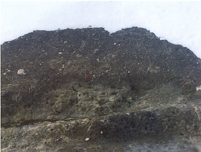
March 31, 2020- Seepage Area
