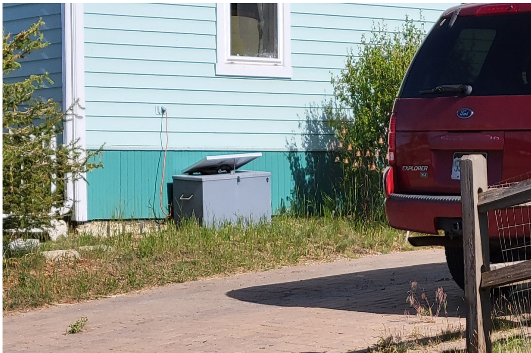
Photo 8. Monitor station at Carl Poch's residence in Cripple Creek, west of Schist Island.
