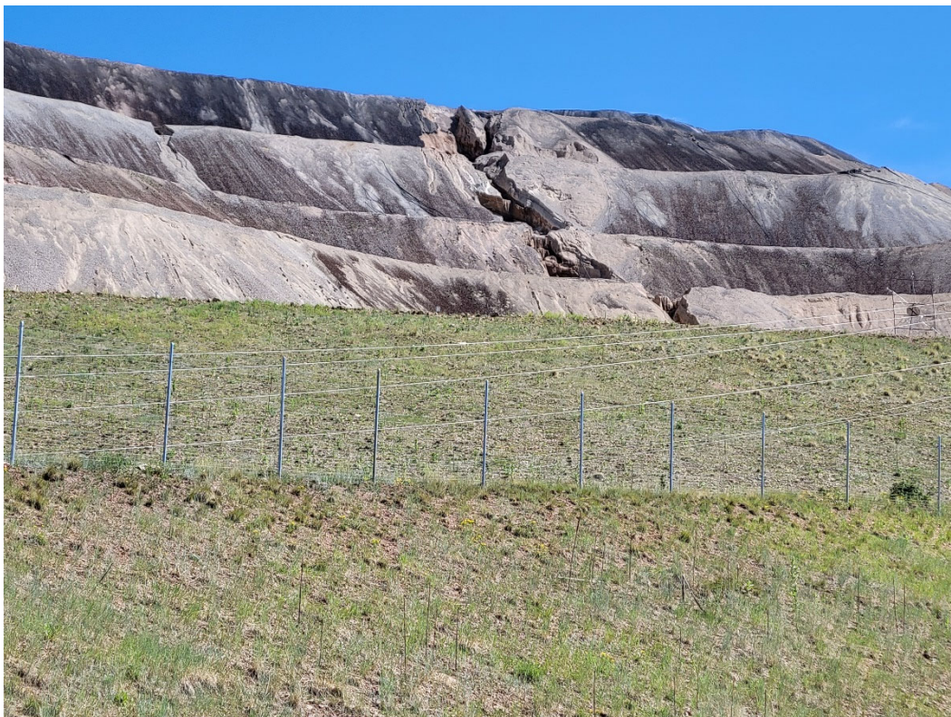
Photo 14. VLF-Phase 5 washout observed by Division, after closeout of inspection.
