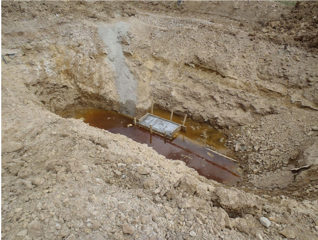
Photo 9. Temporary fix for leaking waterline along toe of ECOSA.
