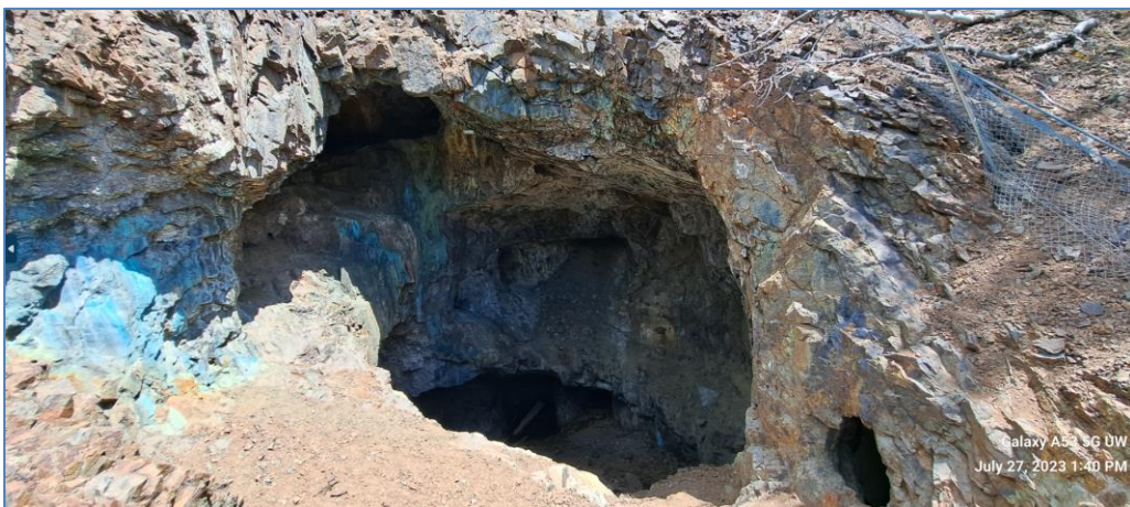
Figure 16: Large daylighted stope. You can see downed fence. Size is ~30 feet wide by unknown depth. Location E on the map.
