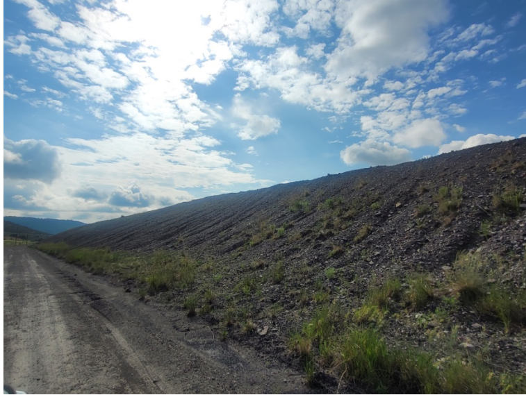
North Facing Side of the DWDA #2
