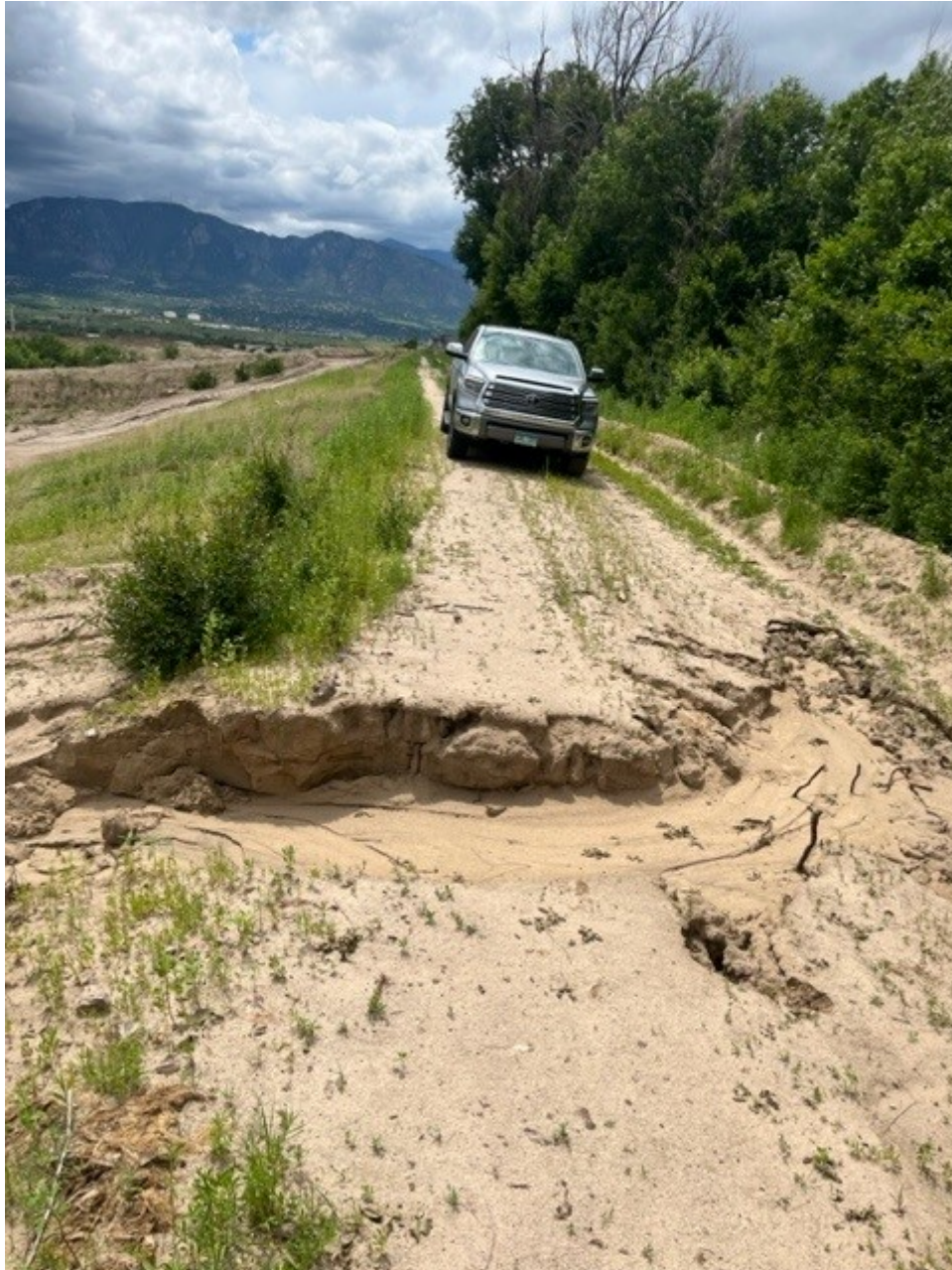
Photo 2. Erosion Gully Traversing the Ditch Road.
