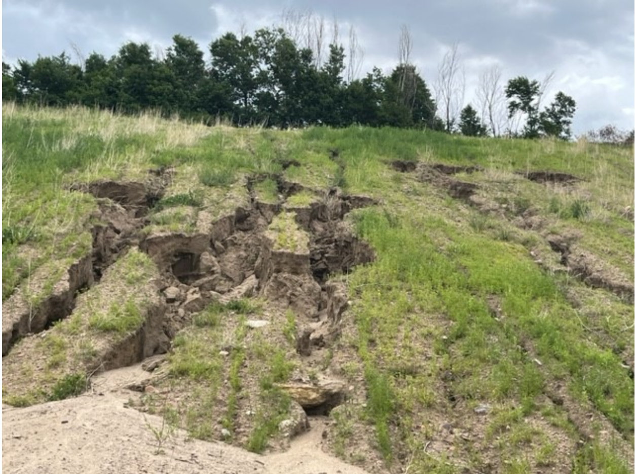
Photo 4. Erosion gullies in central area of buttress in June
