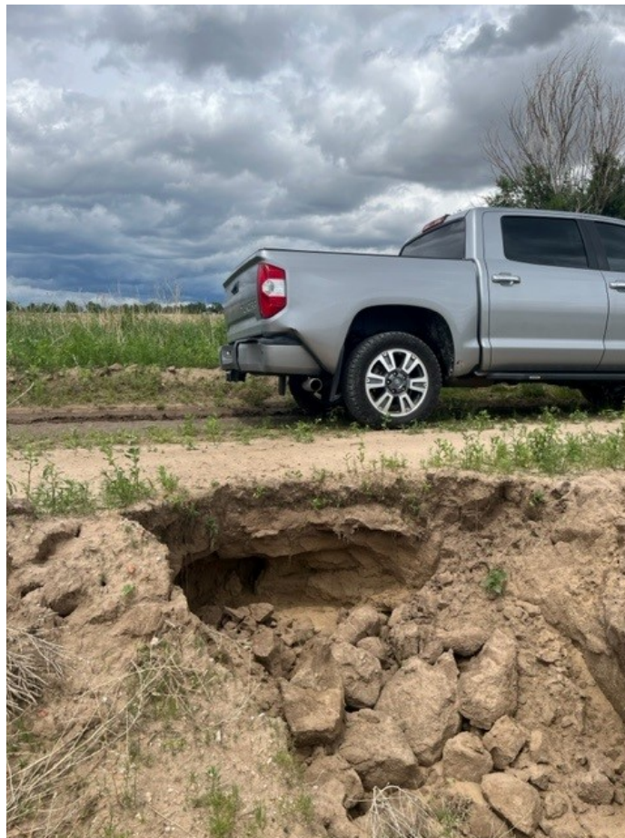
Photo 1. Berm Road Undermined due to Slope's Erosion Gully
