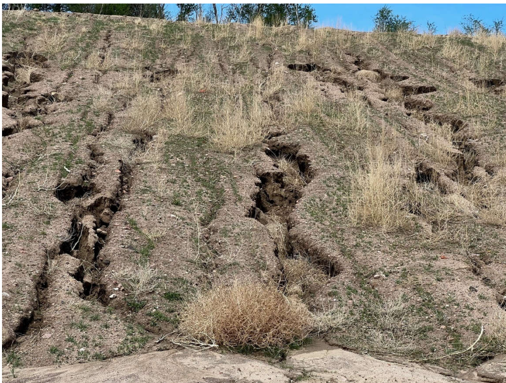
Photo 6. Erosion gullies in central area of butress
