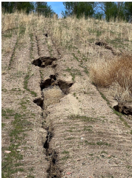
Photo 2. Erosion gullies near west end of buttress
