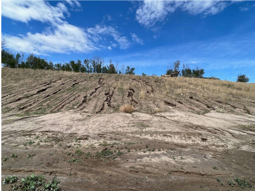
Photo 5. Erosion gullies in central area of butress
