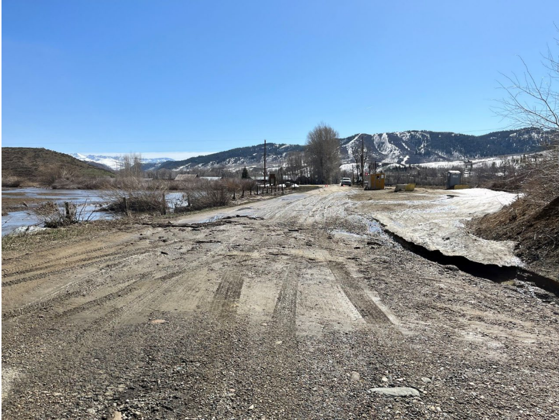
Photo 3: View east of CR62, scale and scale house are visible to the south. Road shows erosional damage from recent flooding.
