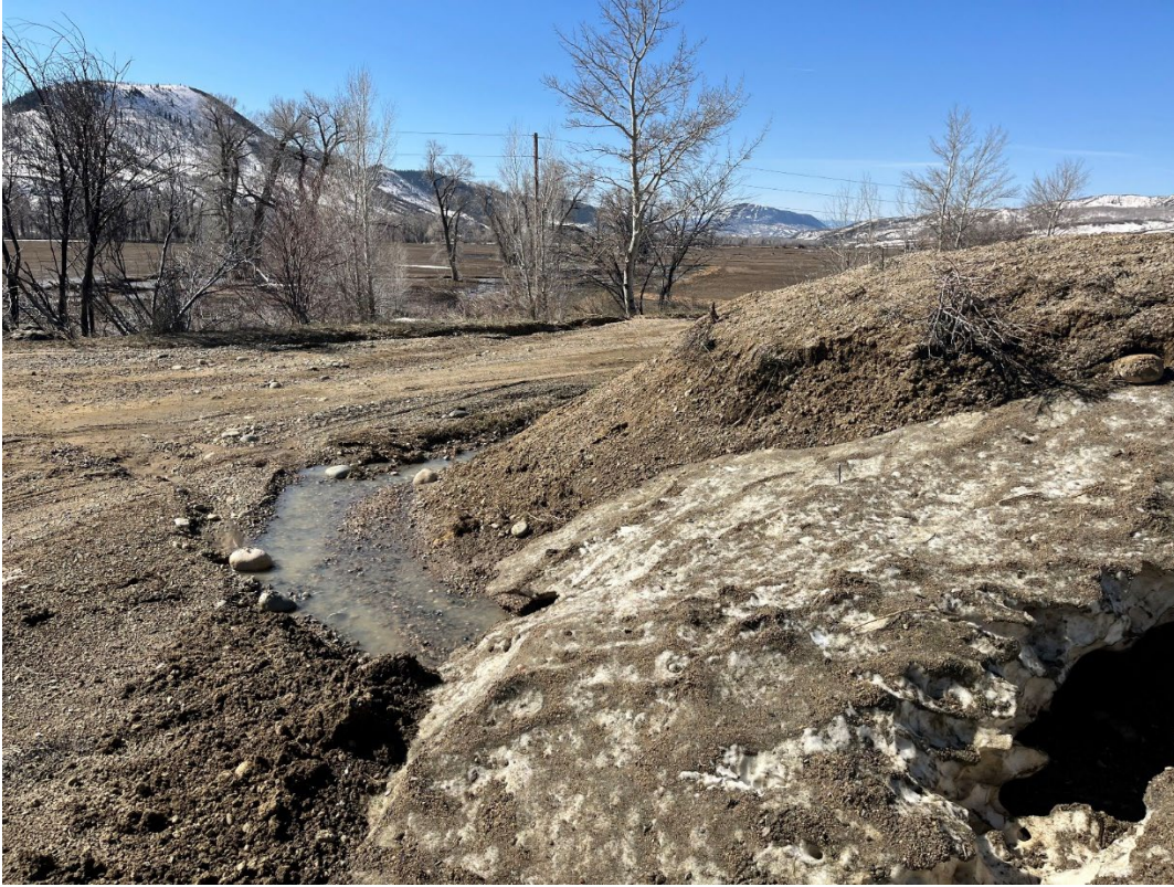
Photo 7: Water is flowing through the dam surrounding the sediment pond and draining to a ditch along CR62.
