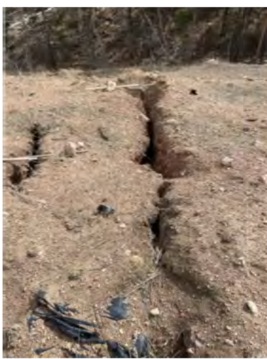
5. Cracks monitored on slopes
