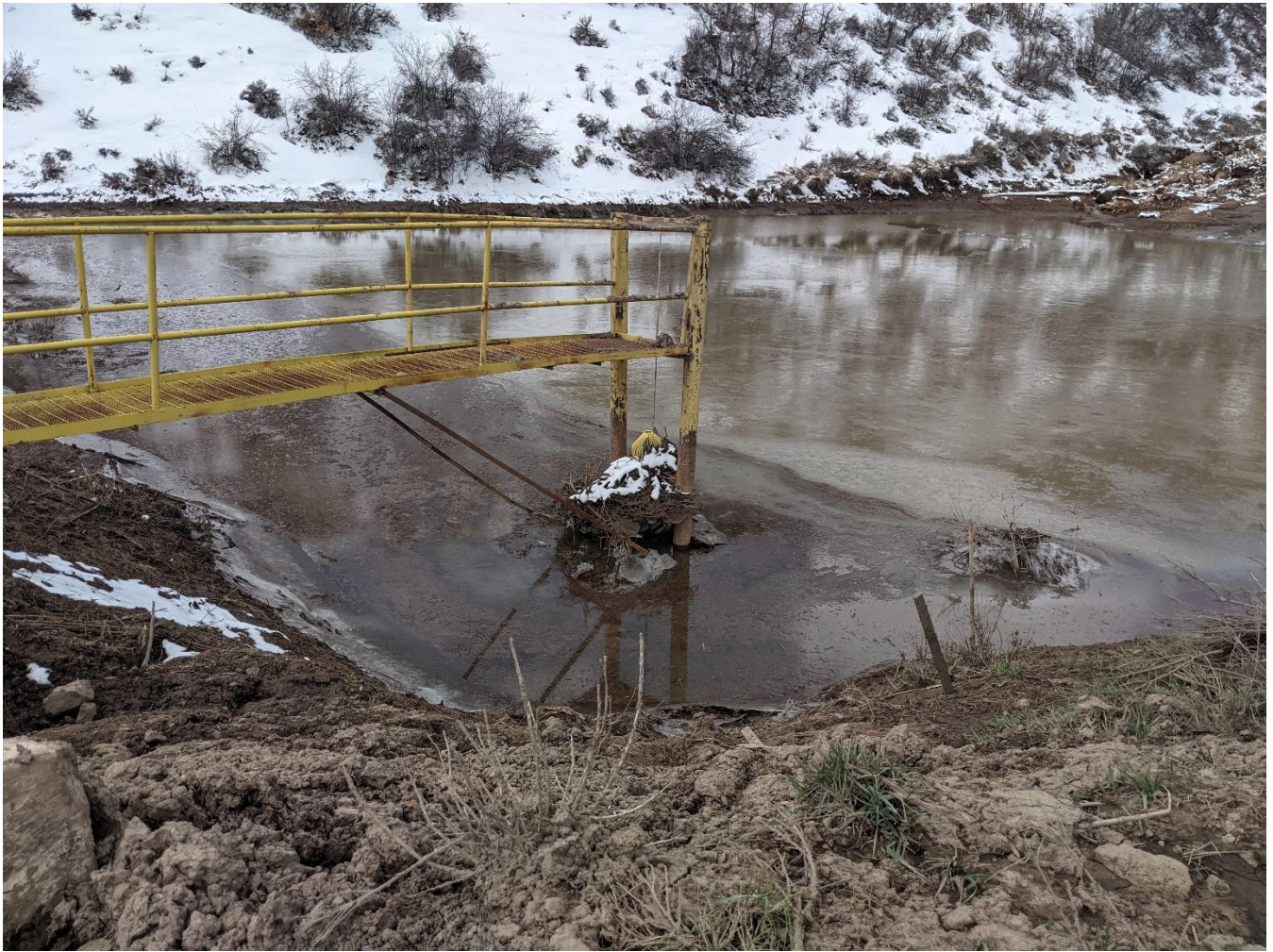
Debris froze on trash rack of Prospect Pond spillway.
