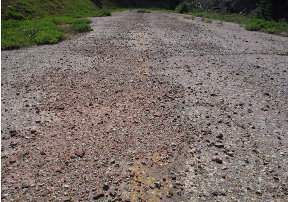
5ST1484.1, Old Colorado State Highway 91 Loop, remaining pavement (F1), view to east.
